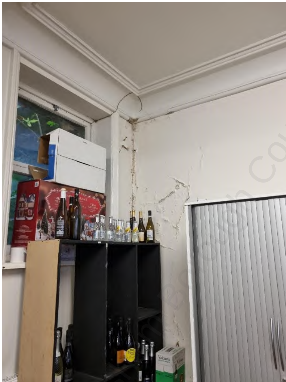
Photo 18: Water damage caused by plant ingress to plasterwork in south west corner of room G.012, ground floor of southern wing
