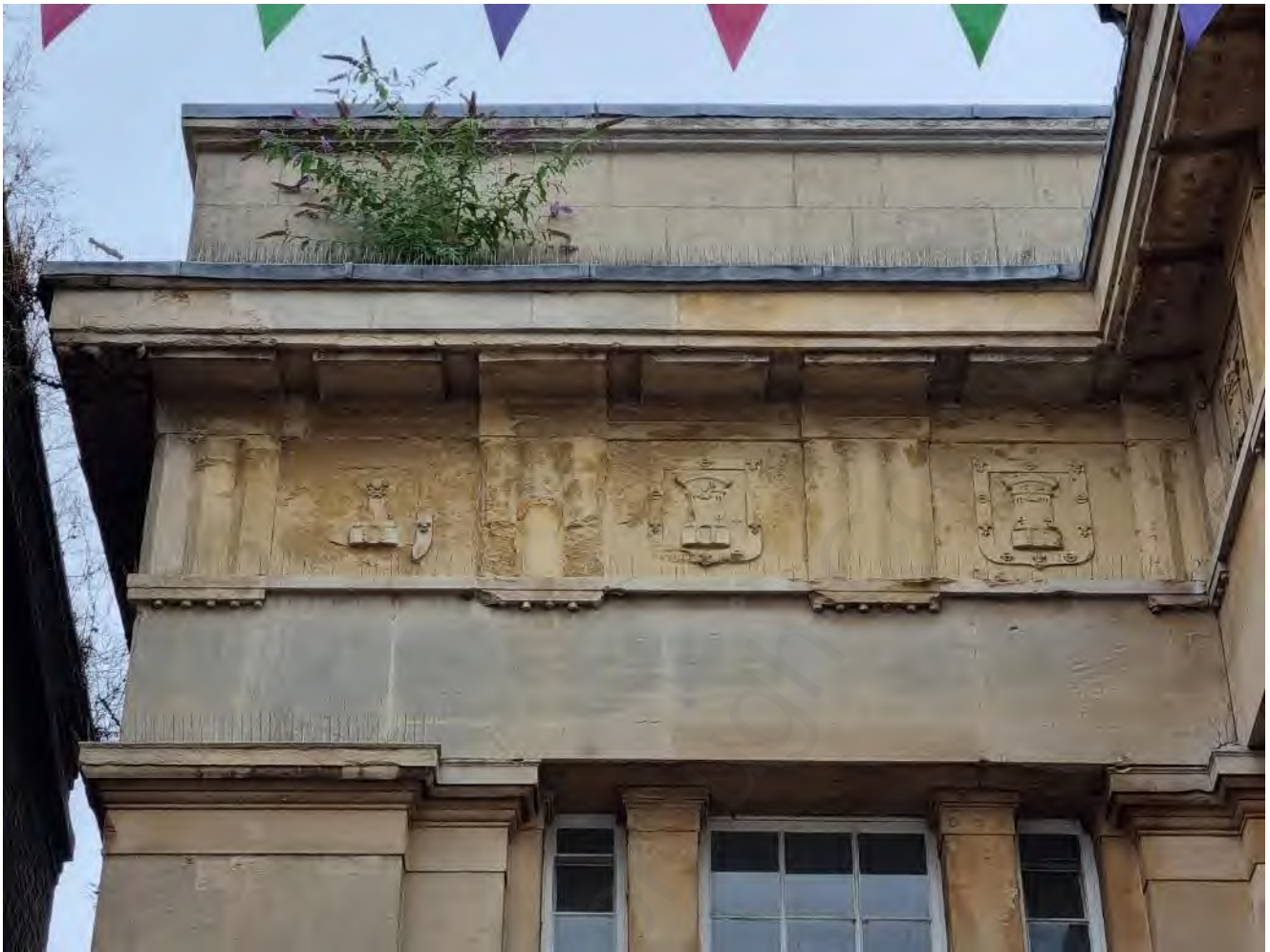
Photo 11: Detail of plant growth from masonry of western elevation
