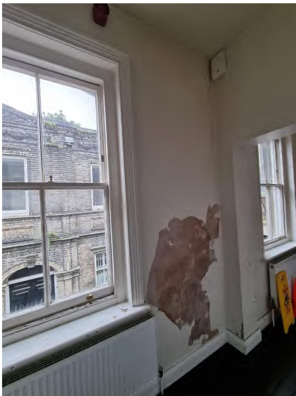
Photo 13: Damage to decorative finish of wall plaster, Room 1.011 (first floor corridor, northern wing)
