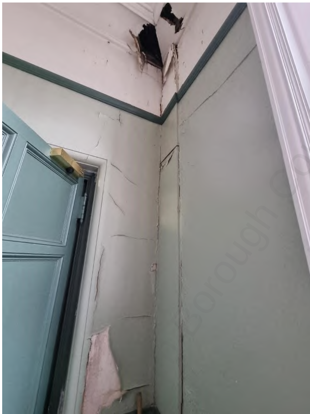
Photo 17: Broken coving and water damage to surrounding plasterwork, north west corner of lobby/stair core Room 1.018 and G.013 in southern wing resulting from damaged internal drainage
