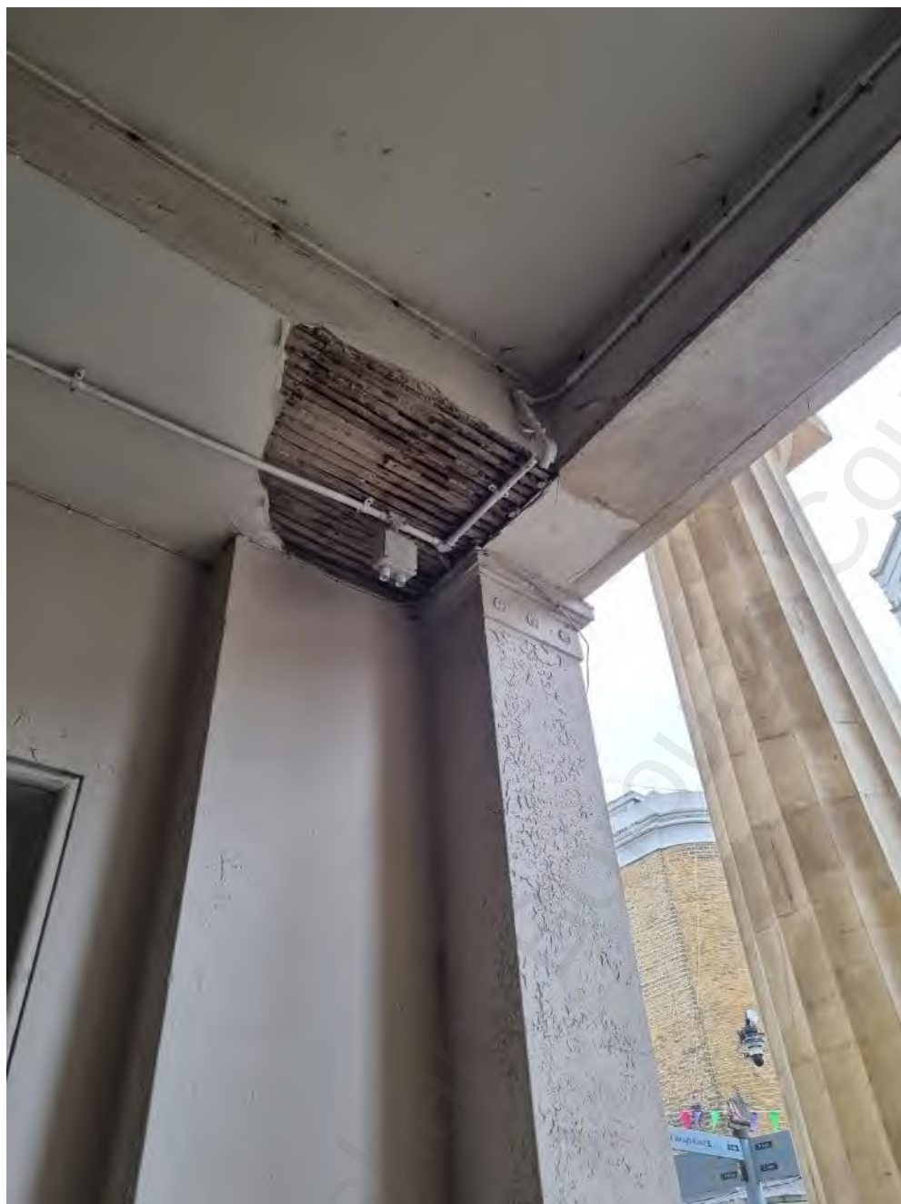
Photo 10: Damage to soffit of undercroft, south west corner adjacent to portico
