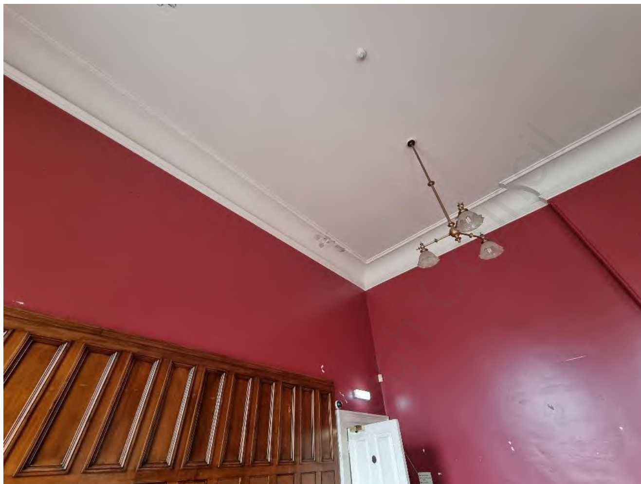
Photo 12: Damage to coving and plasterwork, south east corner Room 1.006 (Old Court Room)
