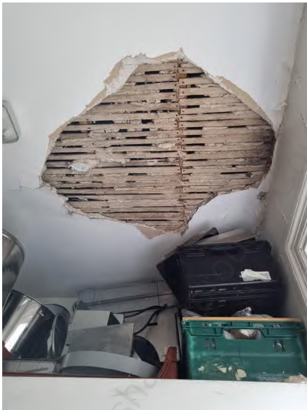
Photo 14: Missing plaster exposing laths to ceiling of Room 1.014, south east corner (first floor storage room, northern wing)
