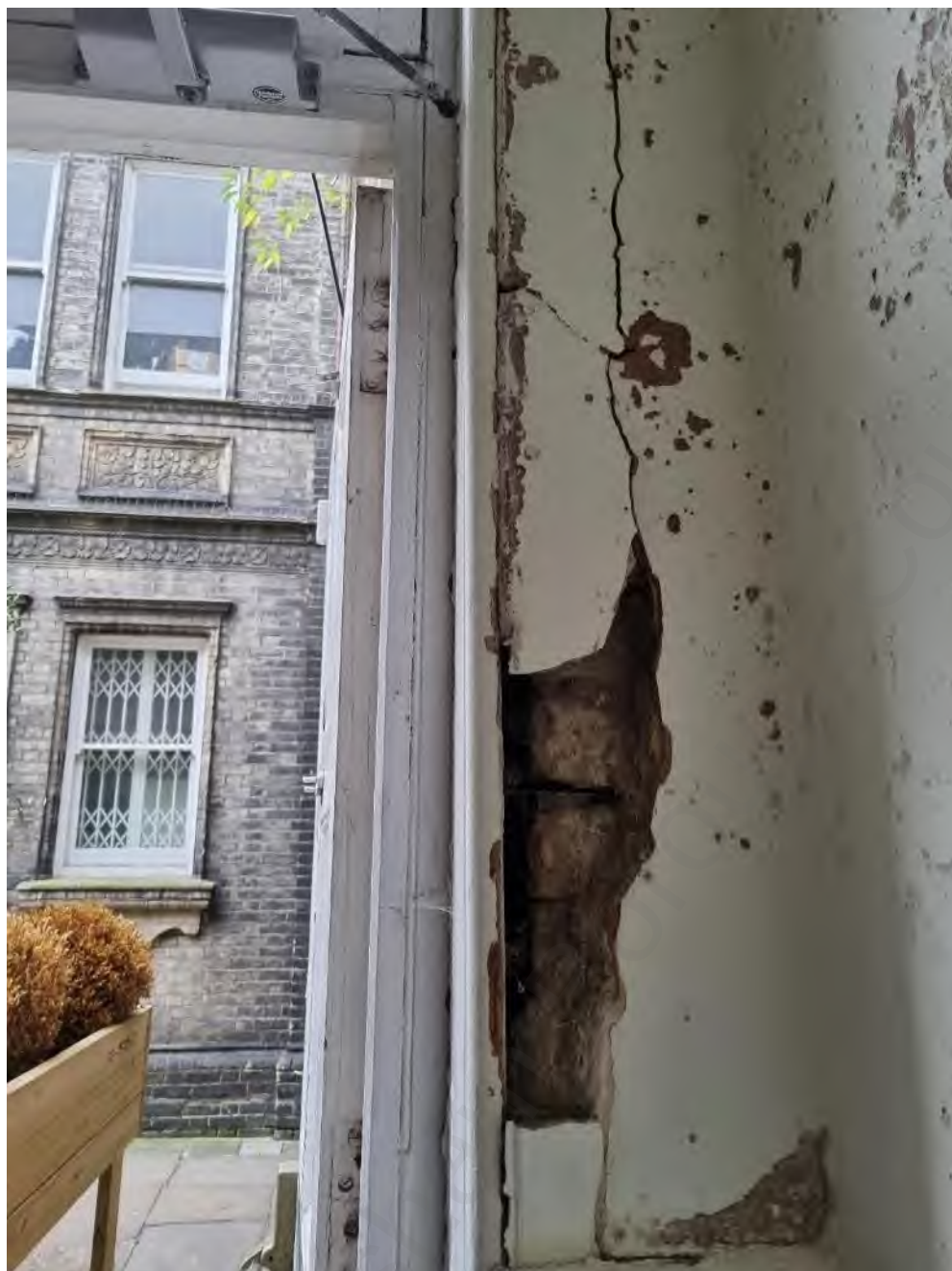
Photo 16: Damaged and missing plasterwork exposing the underlying brick fabric to west of exterior doorframe, G.027 ground floor of northern wing
