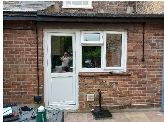
The unauthorised door and window
