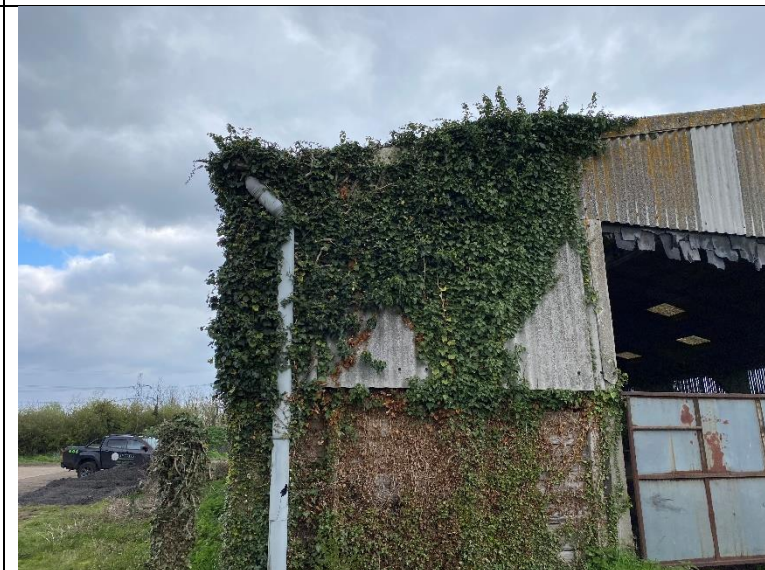
Figure 3 Dense ivy on the north-western corner of B1.
