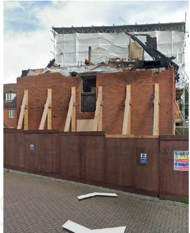
Fig 4 Fire damage to the Side Elevation of No. 104.
