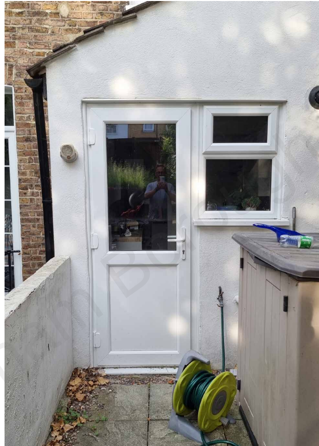
02. Looking at the current white UPVC door and side window requested to be replaced.
