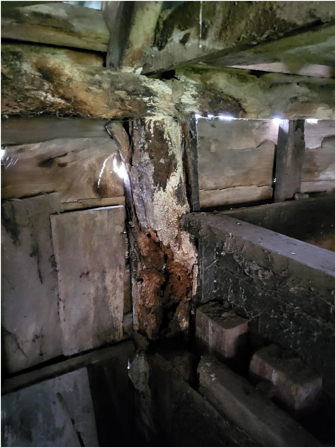
Photograph 5 - Extensive rot to side post in west wall - Grid 5
