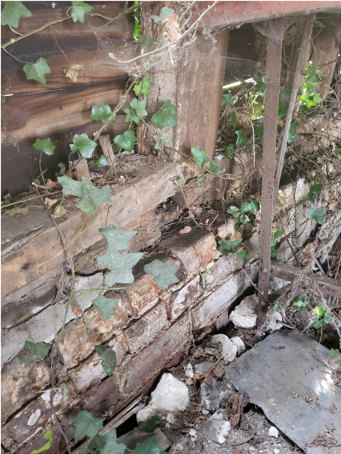
Photograph 3 - Rotten sole plate to south plinth and wall lean
