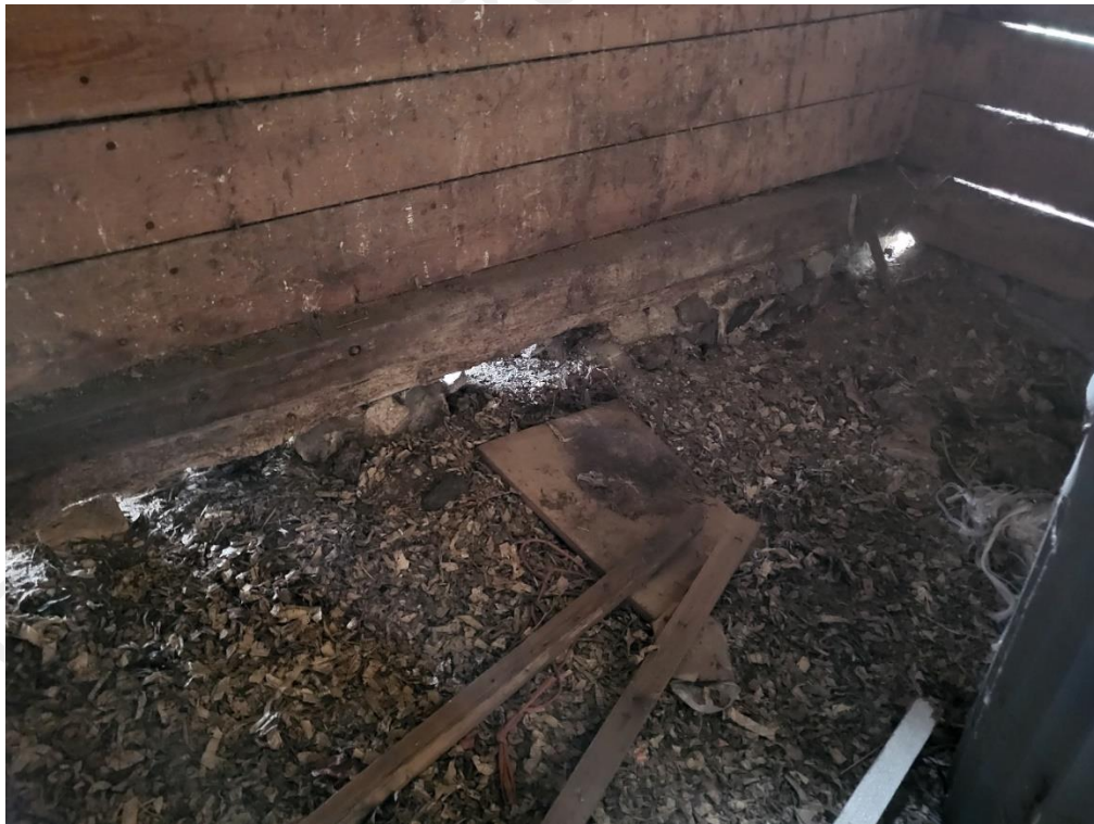
Photograph 9 - Loose and missing plinth to north sole plate
