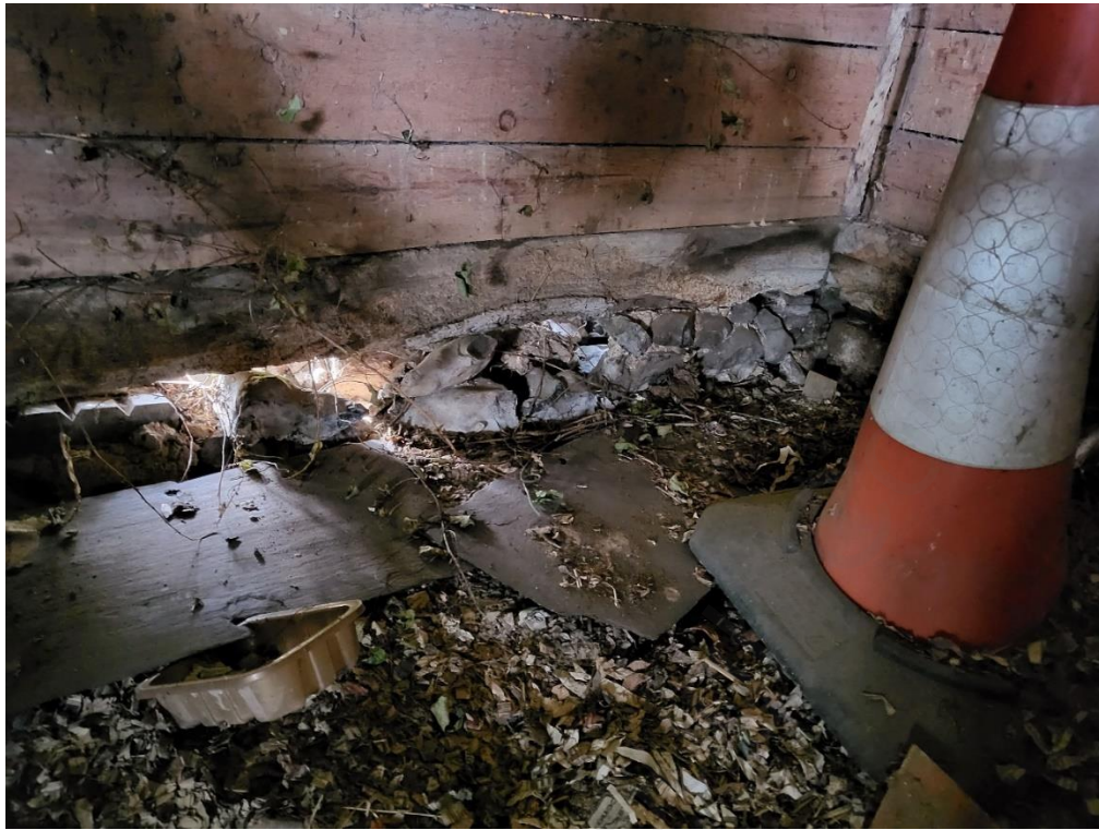
Photograph 8 - Loose and missing plinth to east wall
