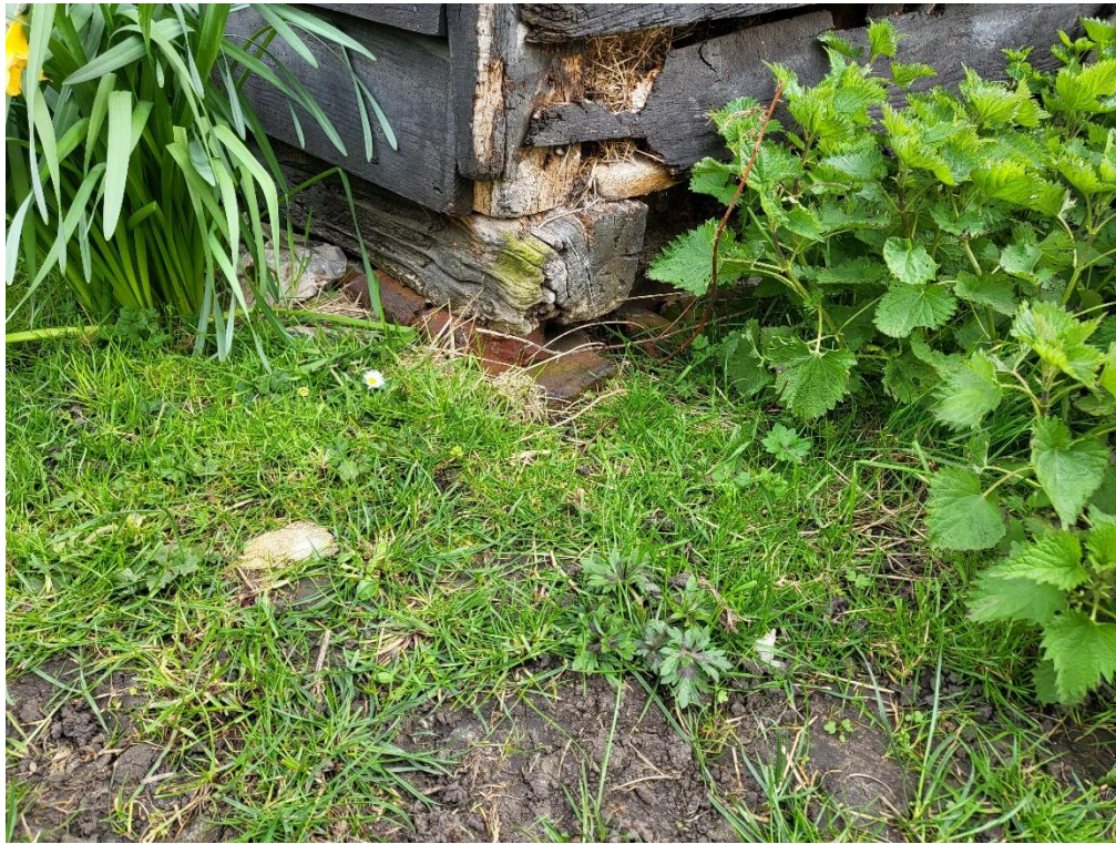
Photograph 23 - Sole plate deterioration in north west corner
