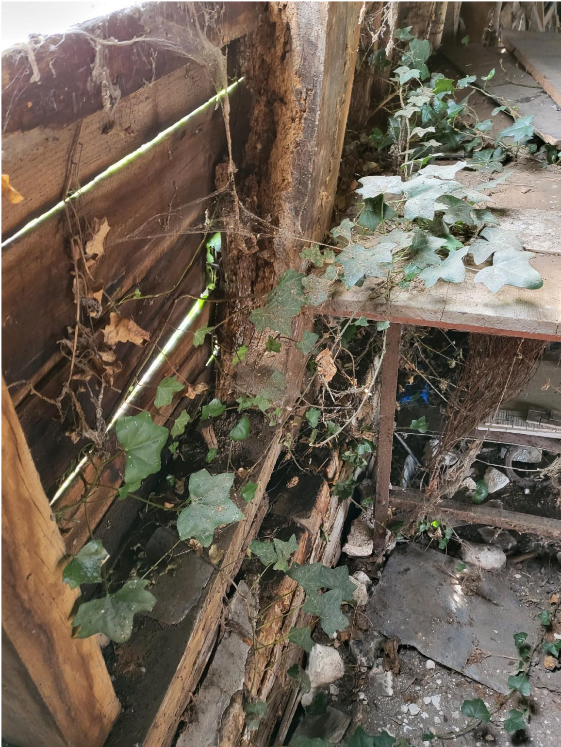
Photograph 2 - Rotten central post to south below window
