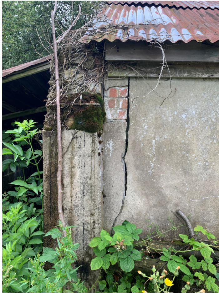
Plate 5 – Section B Grid Reference C2 cracking
