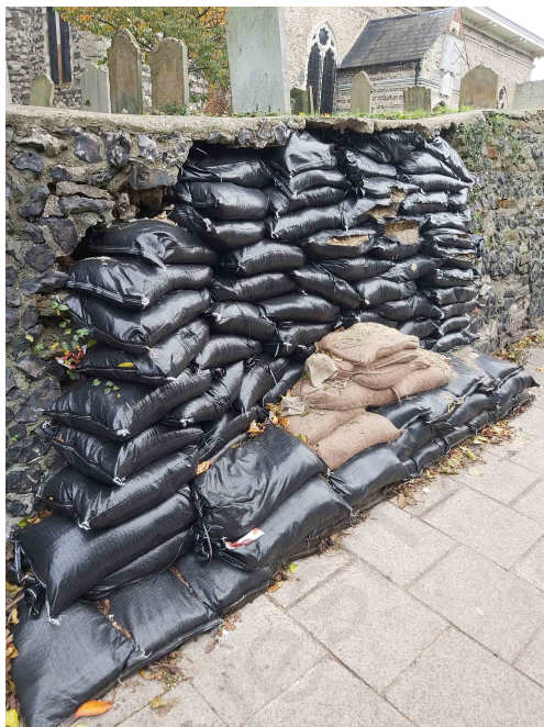
The collapsed section of boundary wall
