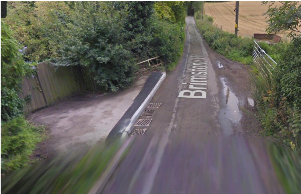
August 2009 Recent highway works which seem to have raised the kerb line to prevent overspill of surface water from flooding the property. Note multiple gully pots that would only be there if there is a severe surface water drainage problem. Gullies also visible in February image.
