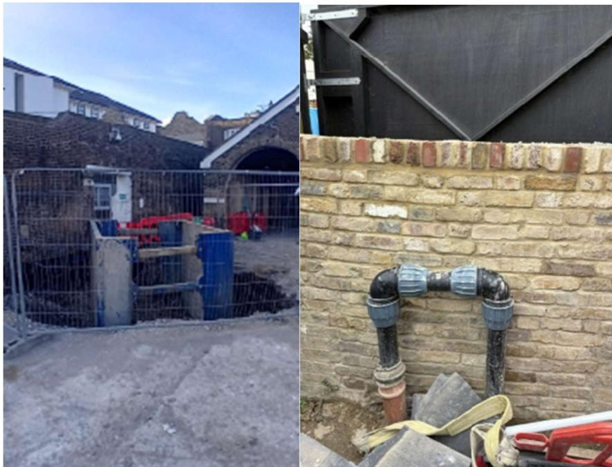
Figure 4-13 Foul water pumping station and break loop.
