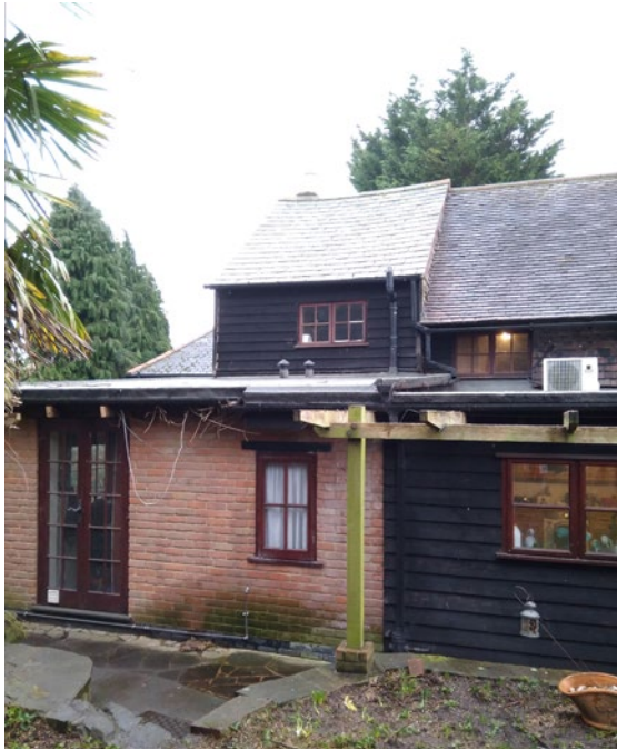
Fig. I I - Photo of the existing poor-quality windows and paint
