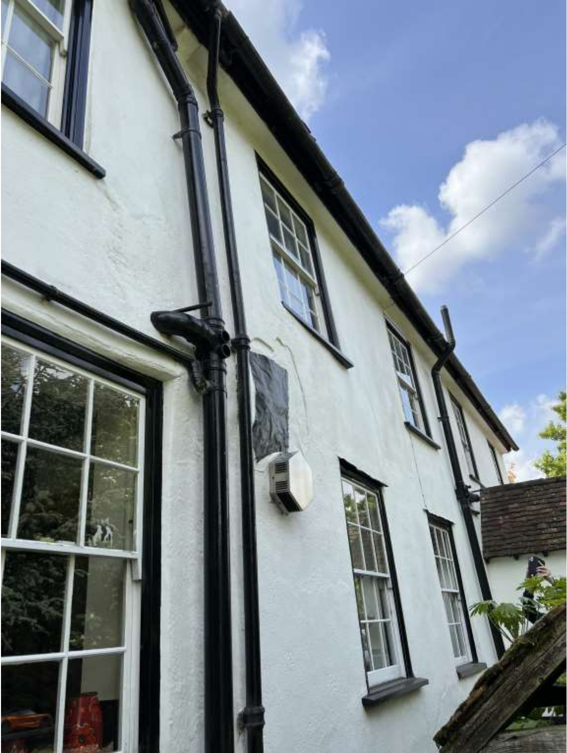
Bulge in external render on north elevation
