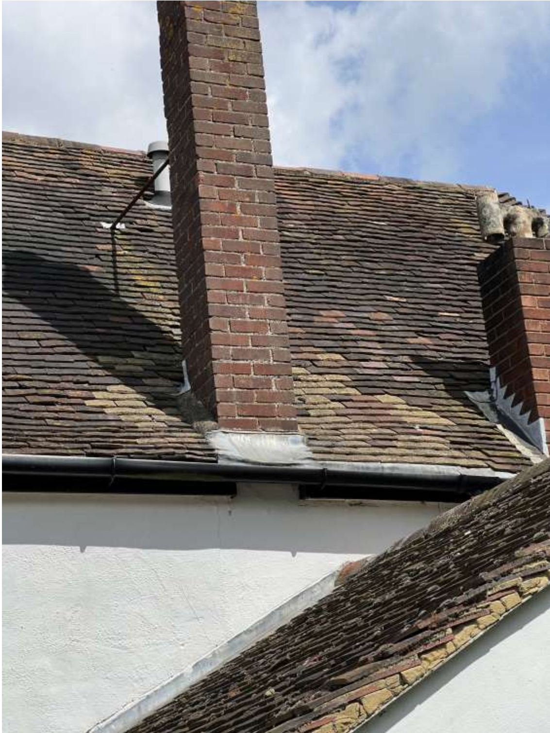
Image showing some mis-matched roof tiles in the main range rear elevation roof-slope and broken flue pot.
