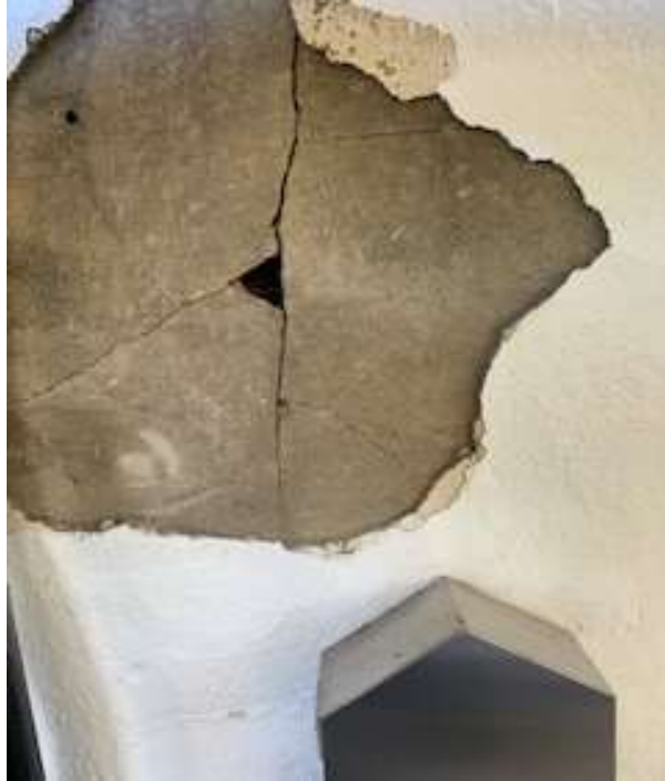
Top coat of render removed where cracking occurred at bulge in north elevation wall, exposing the second layer of ashlar render beneath.
