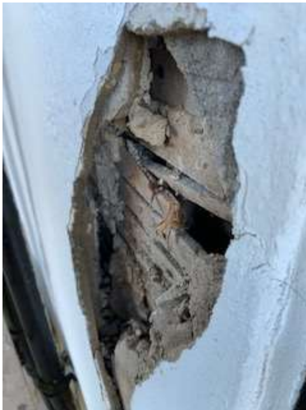
Inspection hole extended to the softwood laths showing the layers of render.
