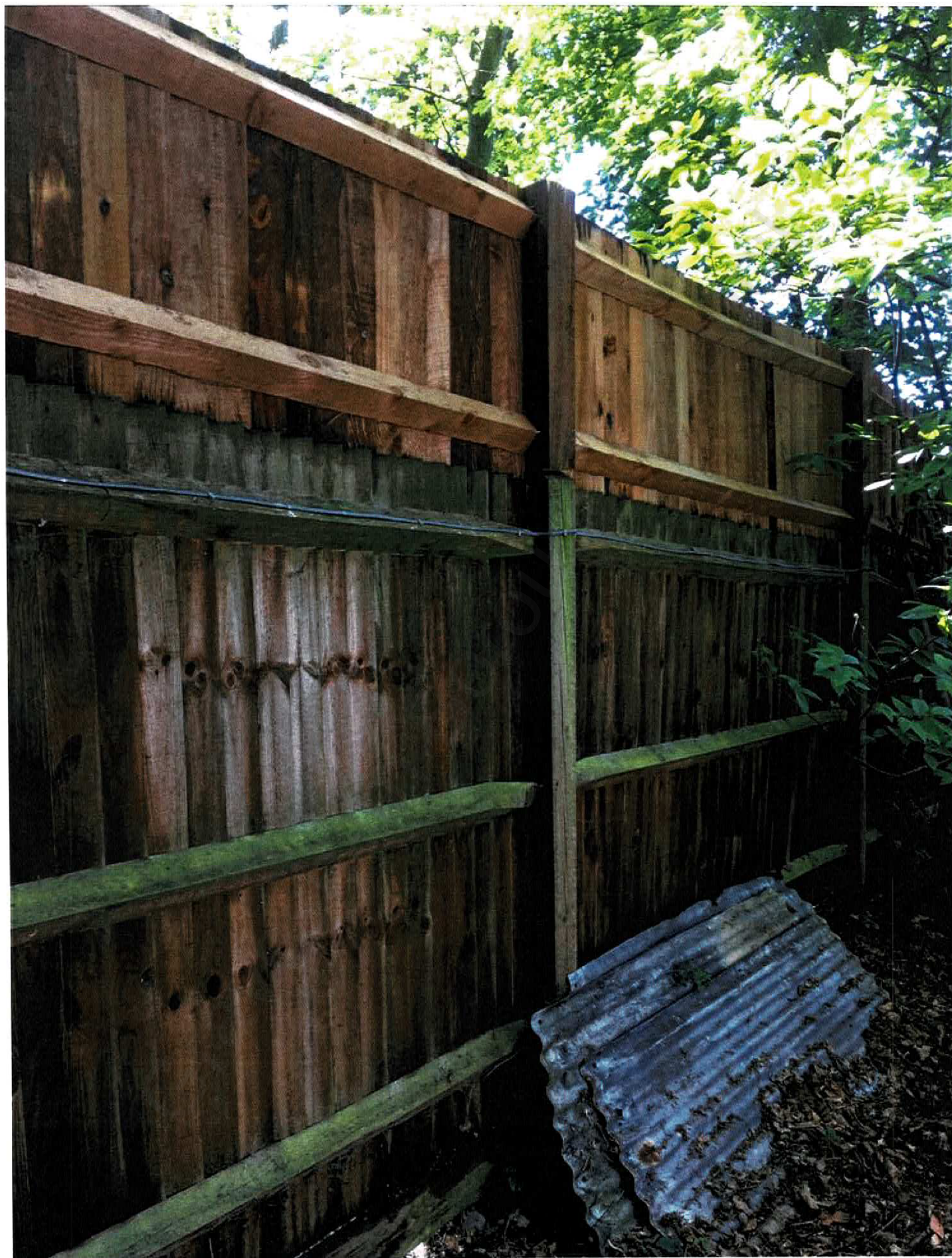
(E) CABLE SECURED TO THE FENCE LINE BETWEEN 'THE LAND' (TITLE TT134110) & LONG ACRE WHICH SUPPLIES ELECTRICITY TO THE CARAVAN & OUTSIDE LIGHTING -
