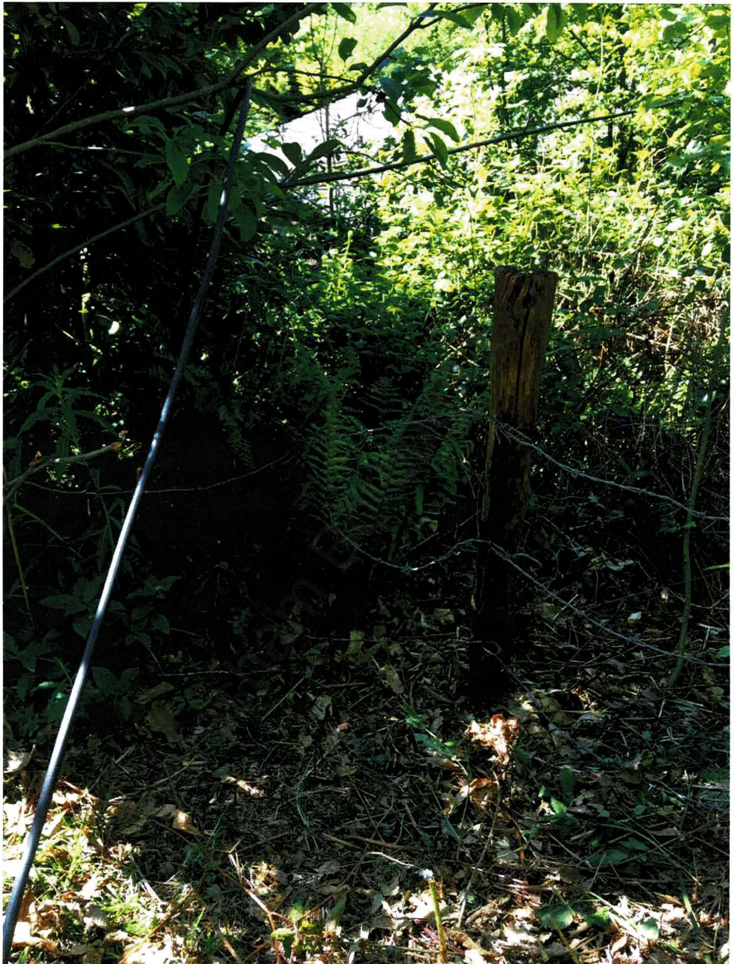
E - ARMOURD CABLE TO THE CARAVAN SUPPLYING ELECTRICITY
