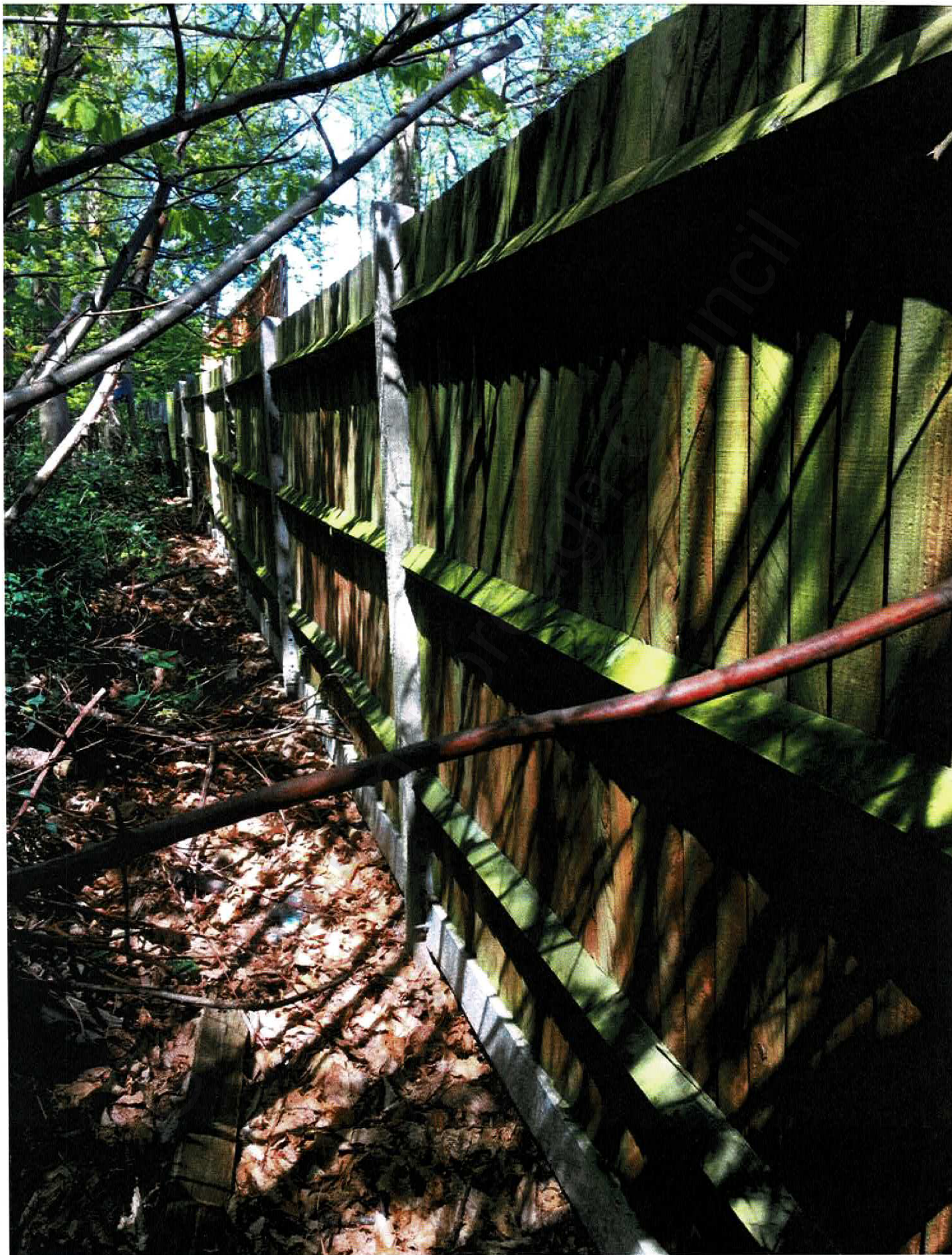
(E) ARMOURD CABLE SUPPLYING AN ELECTRICITY SUPPLY TO THE CARAVAN SITED ON 'THE LAND'
