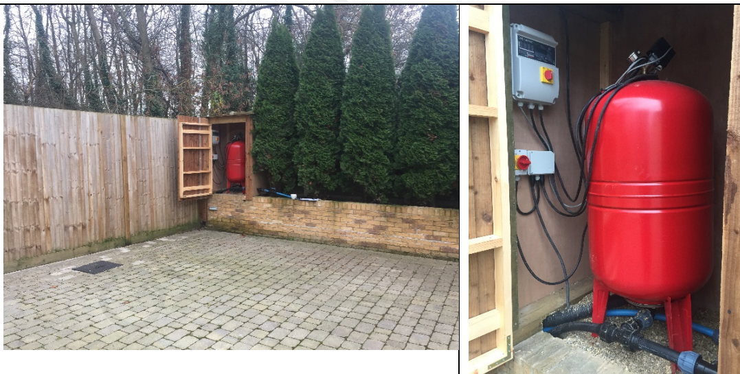
Groundwater Pump in Southeast Corner of Site
