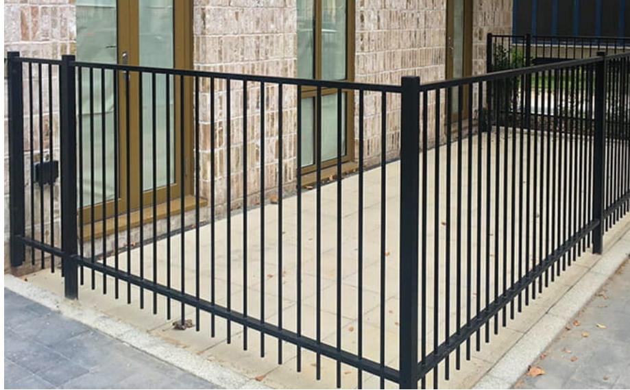
Fig 06 – rear car park area pedestrian safety railing – 21 King Street
