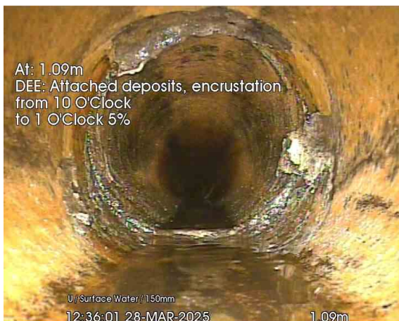
CP01 LAT D_1-09m_123601.jpg, 00:00:29, 1.09 m Attached deposits, encrustation from 10 o'clock to 1 o'clock, 5% cross-sectional area loss
