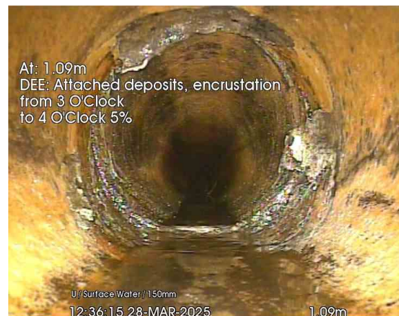
CP01 LAT D_1-09m_123615.jpg, 00:00:31, 1.09 m Attached deposits, encrustation from 3 o'clock to 4 o'clock, 5% cross-sectional area loss
