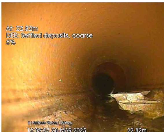
CP01 LAT D_22-82m_123907.jpg, 00:02:02, 22.82 m Settled deposits, coarse, 5% cross-sectional area loss
