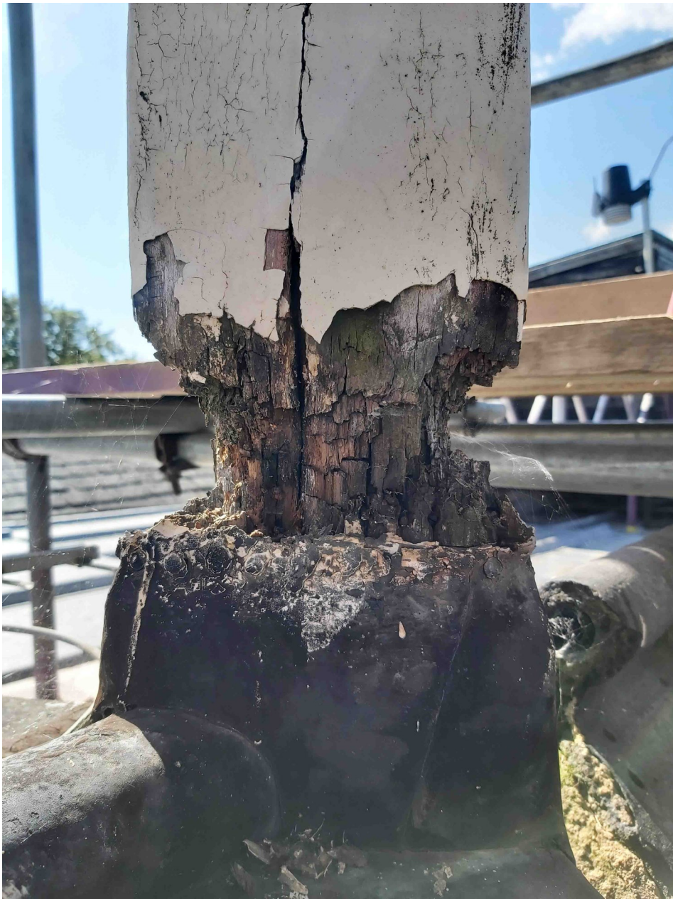
Deterioration on cupola post
