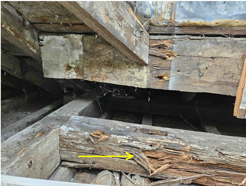
Original base frame showing damaged beam
