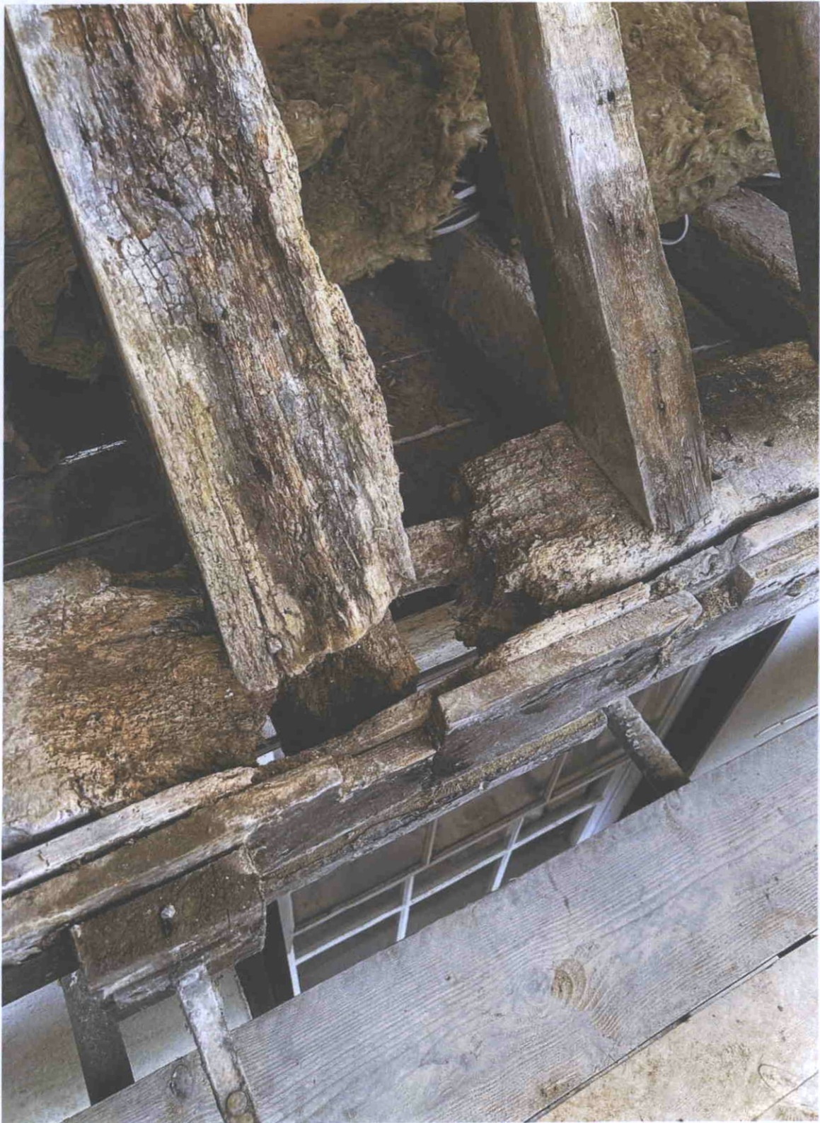
Example of decayed pole-plate on the north elevation
