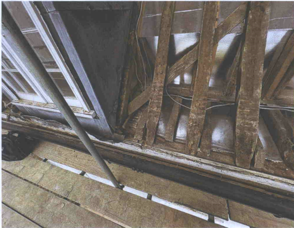
The south elevation roof slope showing short joist ends at bay 2 to the right of the existing dormer.
