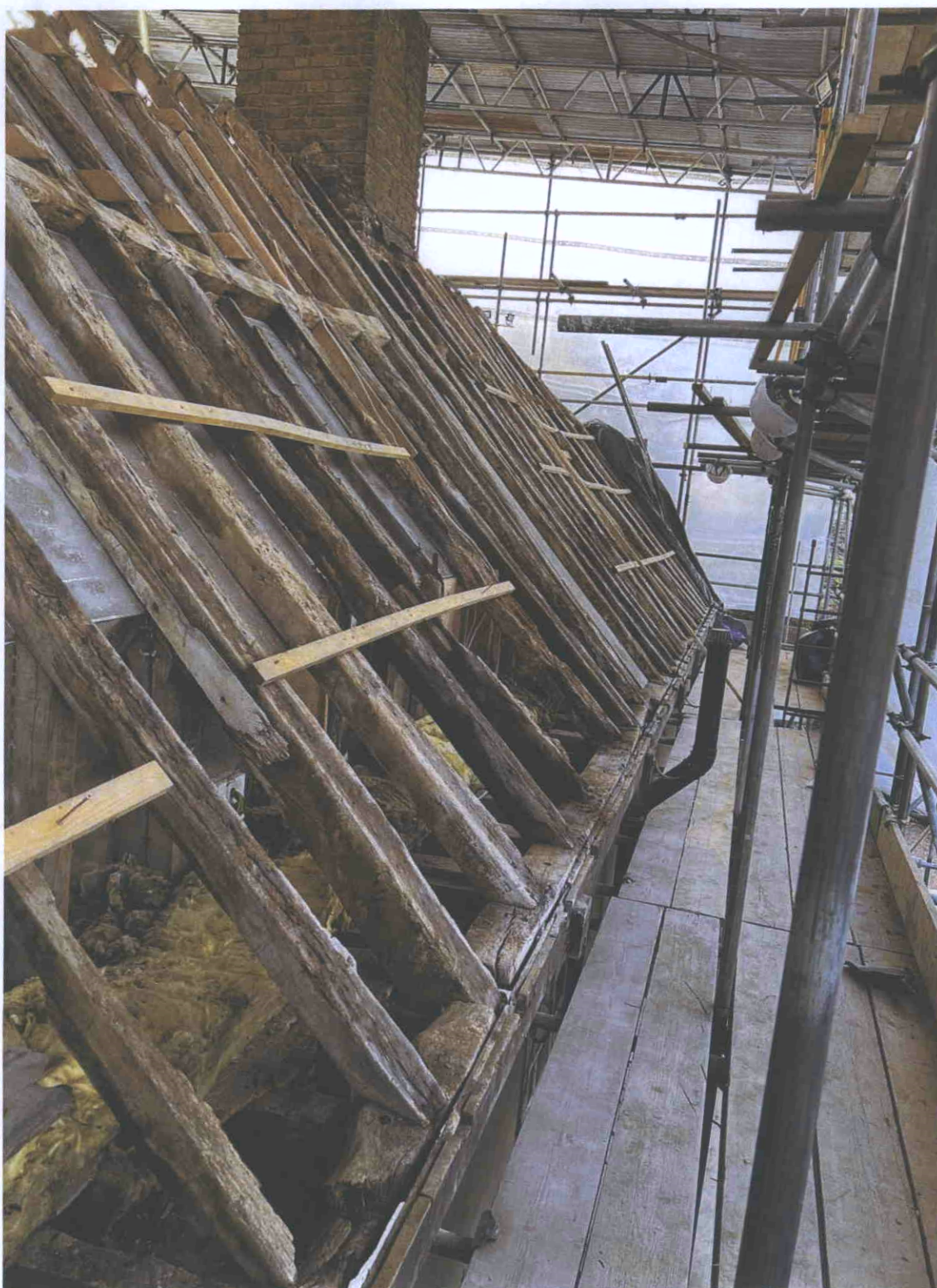
The C17 roof slope of the north (front) elevation showing deflected and decay damaged pole-plates; deflected purlin (bay 3); rafters resting on chimney with no trimmer; and deflected and misaligned rafters.
