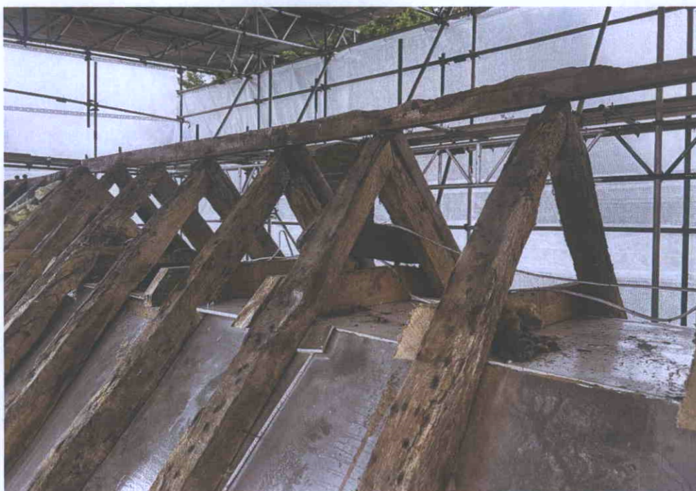
Rafter tops through bay 4 taken from the north roof slope. Note the fake 'ridge board' that had been installed for the now removed furring strips.
