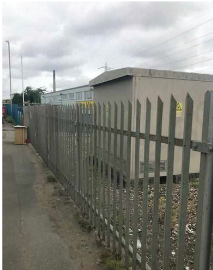
Photo 8: Substation located along the western site boundary off Lower Road.
