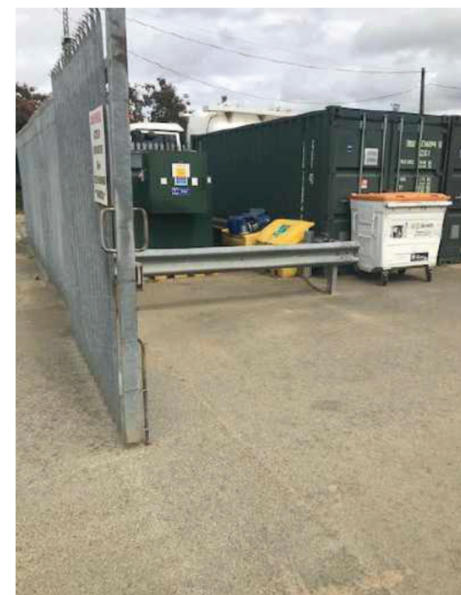
Photo 22: A diesel storage tank, protected and double skinned located in the EA depot.
