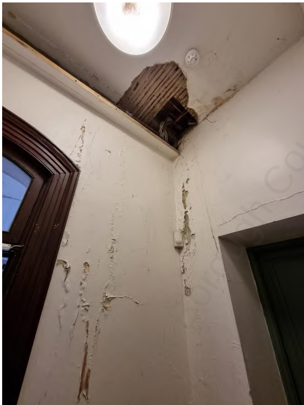
Photo 19: Missing ceiling plaster and water damage to high-level wall plaster in north east corner of lobby G.047, ground floor of southern wing
