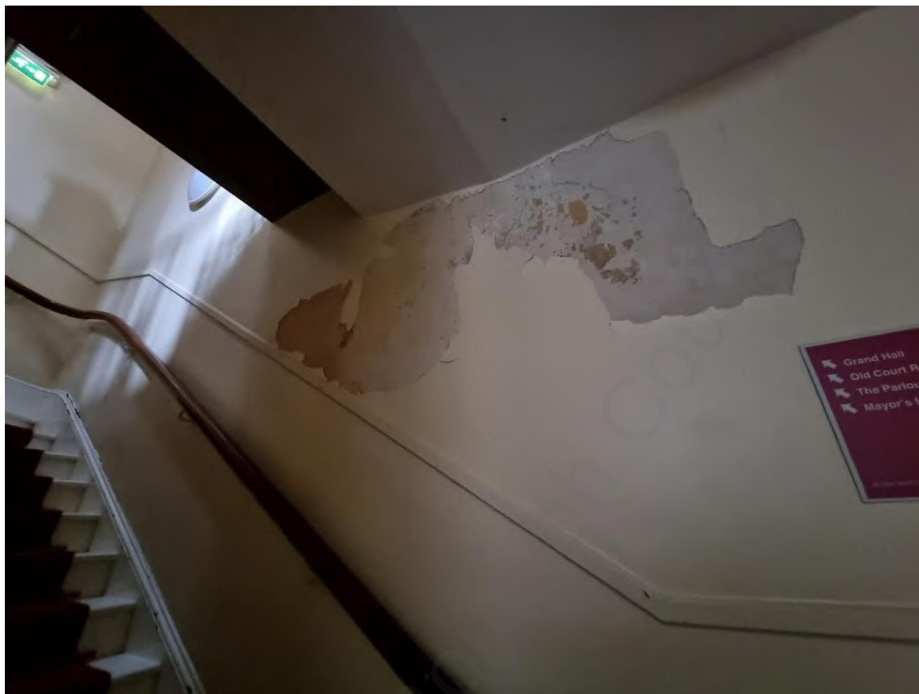
Photo 15: Damaged paintwork within lower stair core G.027, ground floor of northern wing
