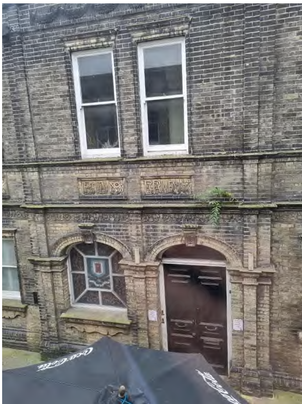
Photo 7: Central bay of southern wing facing south showing plant growth from brickwork.
