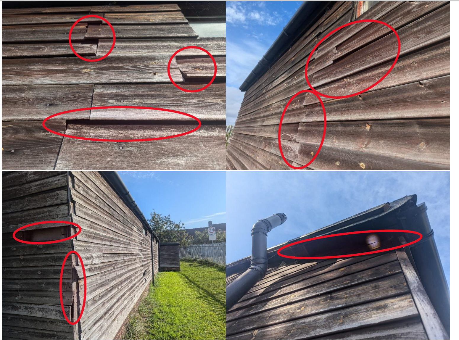
Figure 8: Damage and gaps under timber boarding
