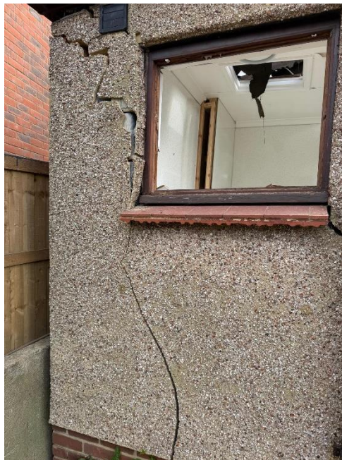
Figure 13. Separation and cracking through the external wall and brickwork, demonstrating structural movement.
