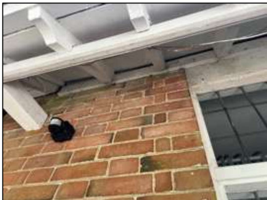
Photograph 5: Gaps at eaves of B1a.
