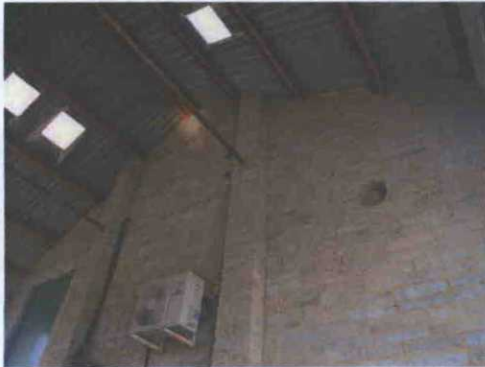
The archway of B2b showing gap at the top
