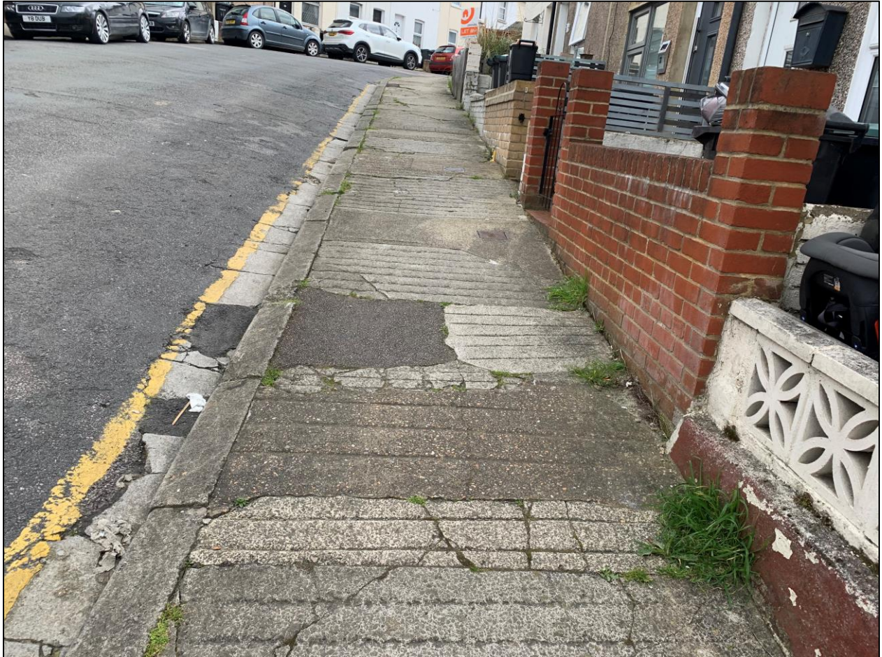
Photo 6: Poorly maintained footways (Hamerton Road)
