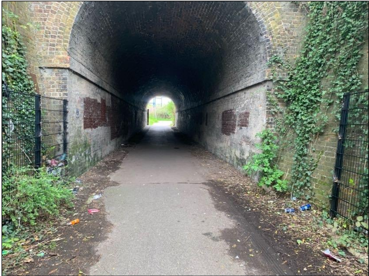
Photo 15: Lack of lighting in and around tunnel
