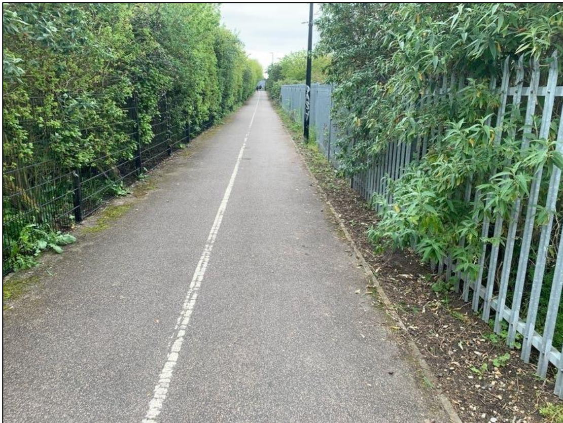
Photo 14: Overgrown vegetation on shared path
