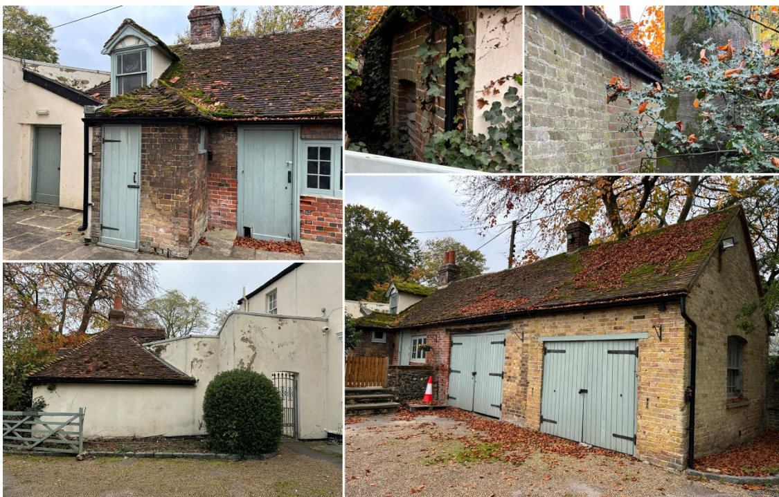
Image 5: Photographs of front outbuilding, highlighting heavily-compromised building fabric (refer to condition report for photographs highlighting internal damage).
