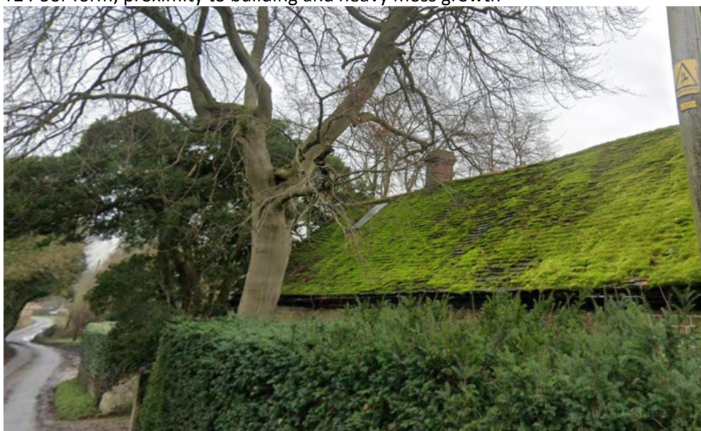
T2 Poor form, proximity to building and heavy moss growth
