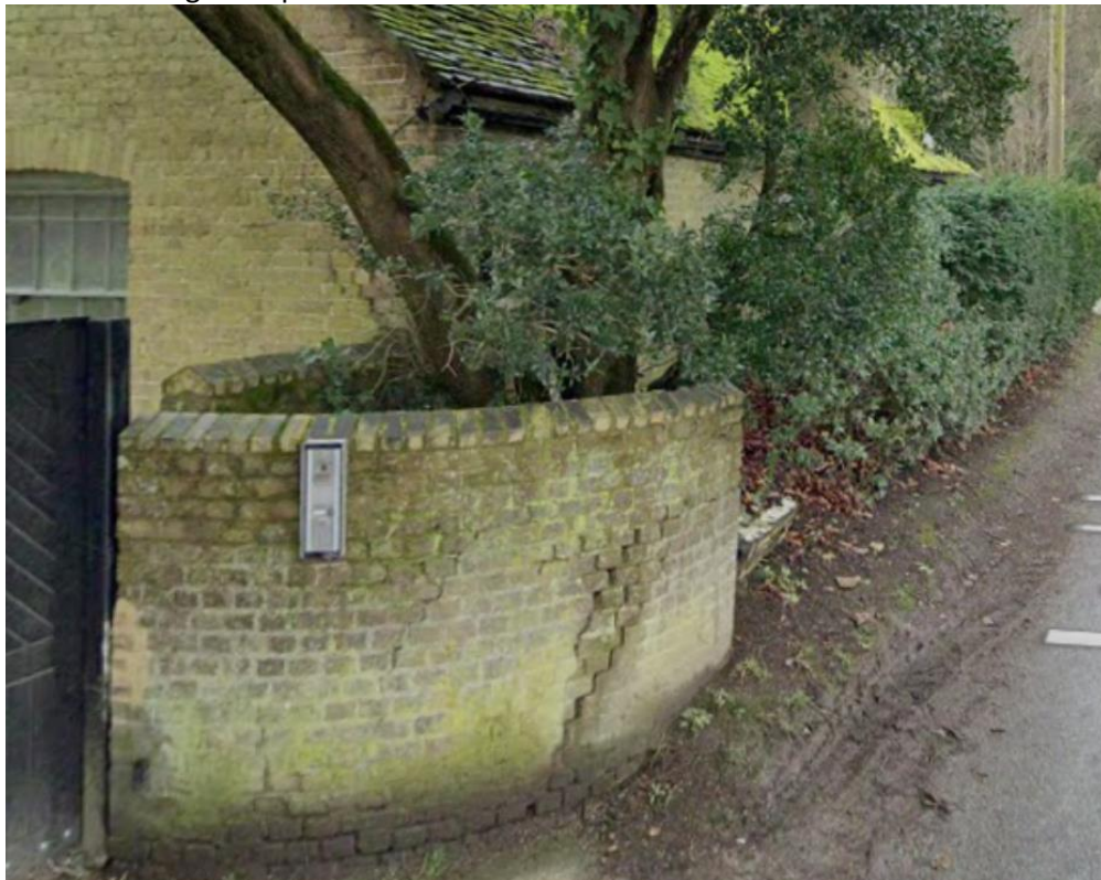
T1 Wall damage and poor form
