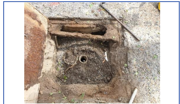
Fill point infrastructure within manhole
