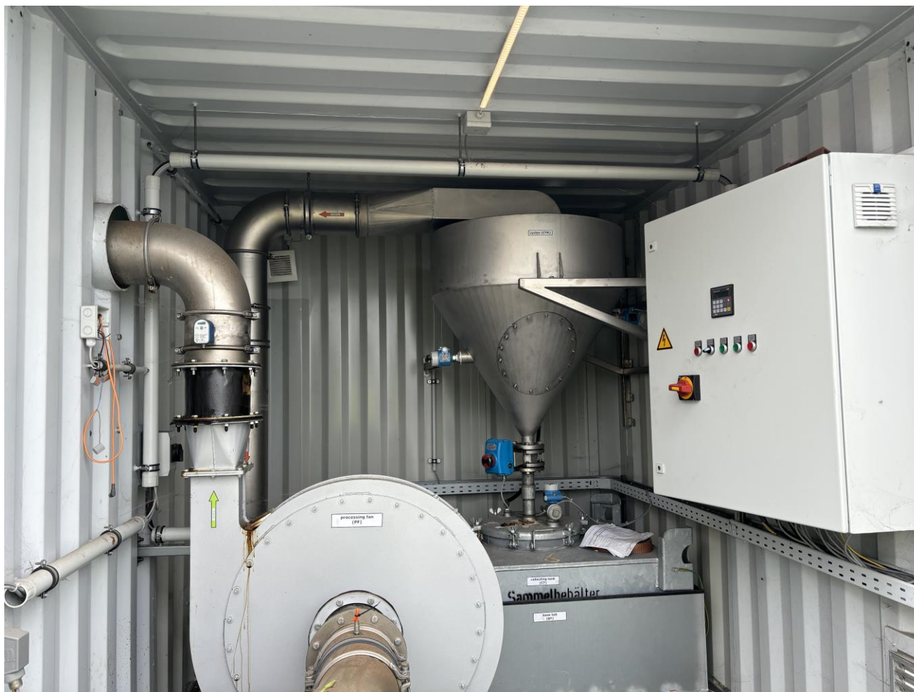
Figure F1 Extraction Fan within the Existing Loading Gantry
