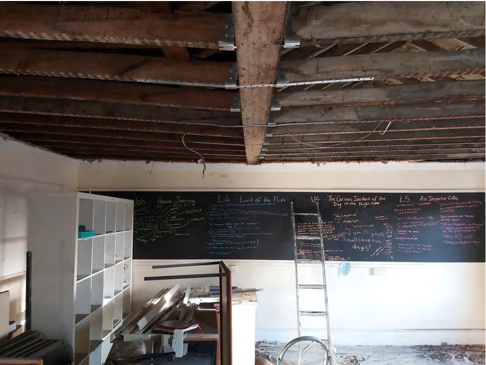
Ceiling of HSFX06 H1 classroom looking east After ceiling came down on the advice of the SE straps were fixed to underside of main beam. Photograph taken 23/11/2022 by CP
