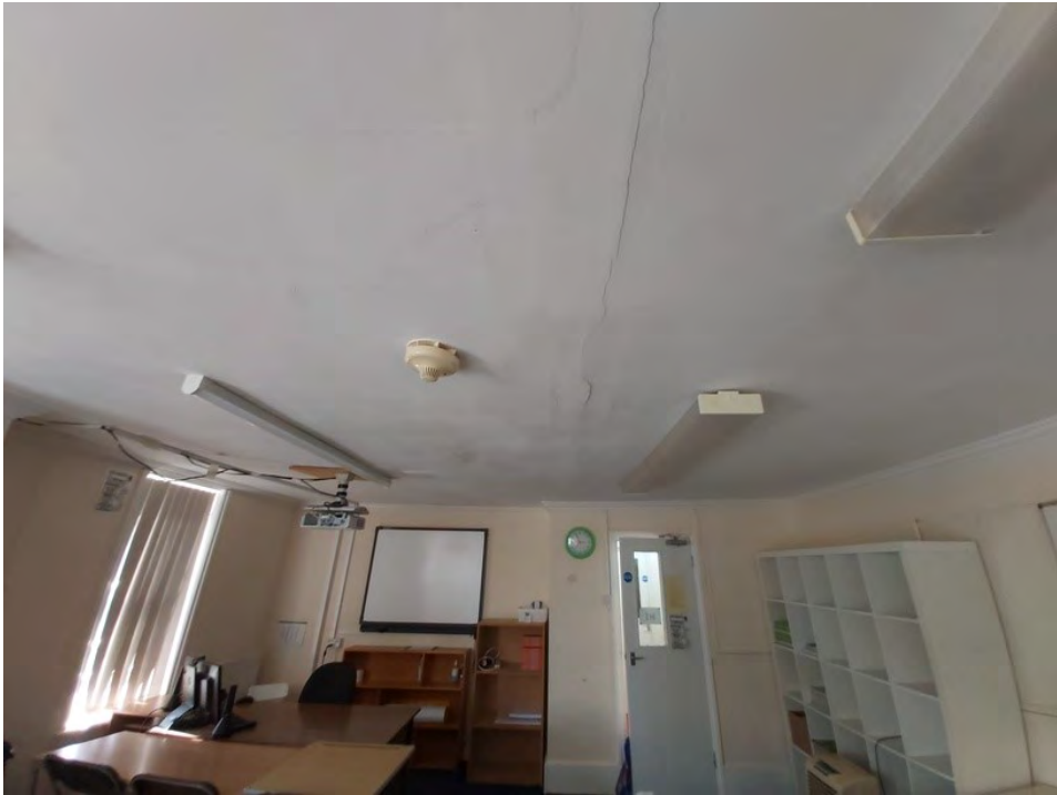
Ceiling of HSFX06 H1 classroom looking west Ceiling shows signs of cracking , sagging and previous repairs. Photograph taken 01/08/2022 by CP
