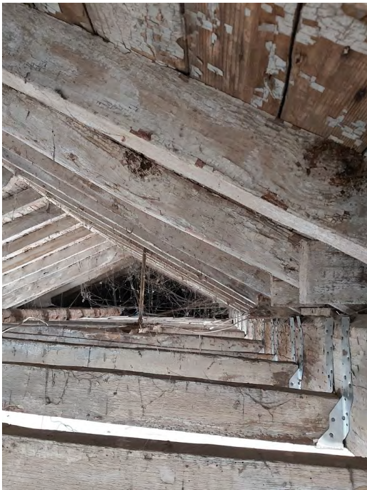
Ceiling of HSFX06 H1 classroom looking east west Sarking boards have been lime washed . Some boards are showing signs of damp ingress Photograph taken 23/11/2022 by CP
