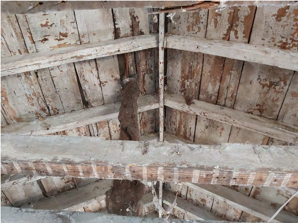
Ceiling of HSF06 H1 classroom looking east west Underside of roof RFX02. Gaps between sarking boards. Some are rotten and damp coming in from above. Photograph taken 23/11/2022 by CP
