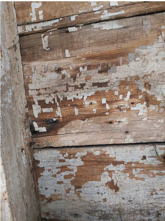
Underside of roof HRFX02 of HSFX06 H1 classroom looking at the sarking boards. Sarking boards showing signs of water ingress coming in from above. Photograph taken 23/11/2022 by CP
