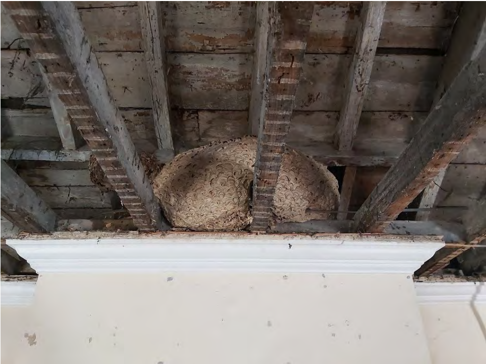
Ceiling of HSF06 H1 Classroom looking south Bee/ wasps nest above fireplace. Photograph taken 23/11/2022 by CP
