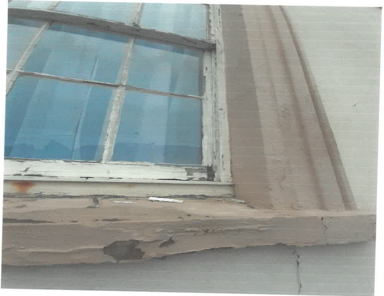
Typical condition of frames and units
