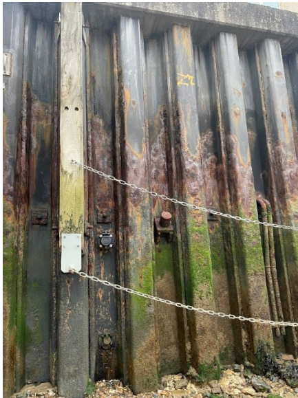
9 - Surface corrosion visual inspection
