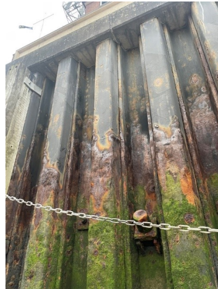
10 - Surface corrosion visual inspection
