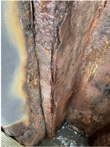
13 - Delamination example before
