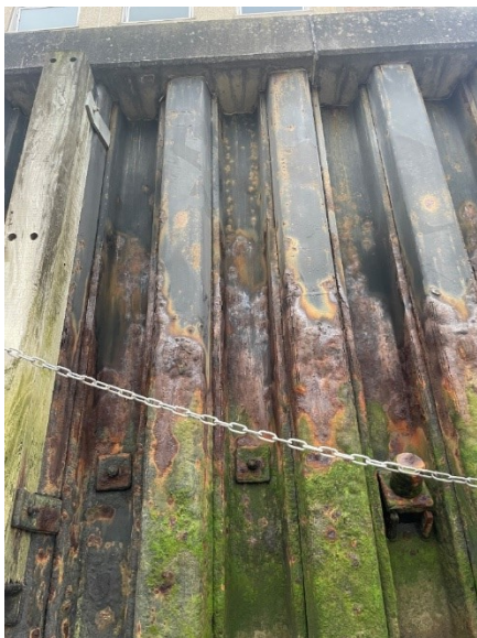
11 - Surface corrosion visual inspection
