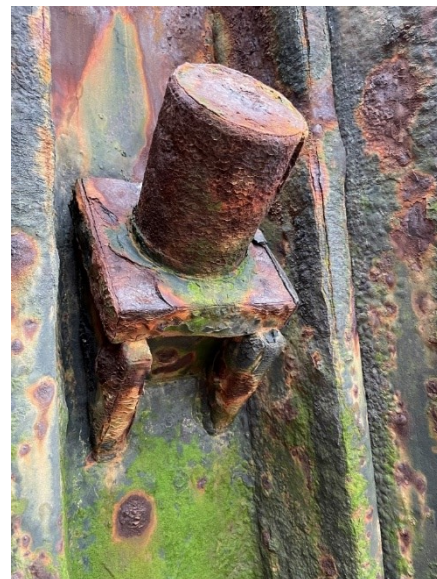
12 – Tie bar and surface corrosion
