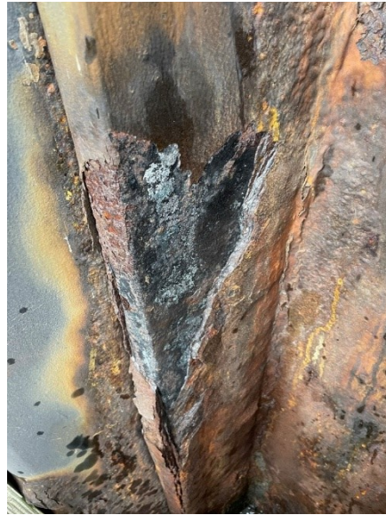
14 - Delamination example after
