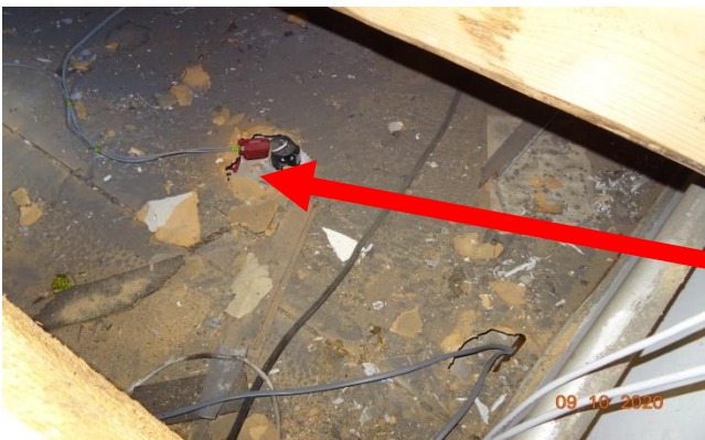
Location Ref 4: Sample TAG/A/S-07- Ceiling Voids To Main Reception And WC - ASBESTOS DETECTED AMOSITE (BROWN ASBESTOS).
