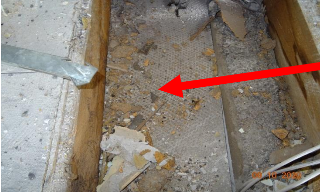
Location Ref 18: Sample TAG/A/S-07- Void To Floor - ASBESTOS DETECTED CHRYSOTILE (WHITE ASBESTOS).
