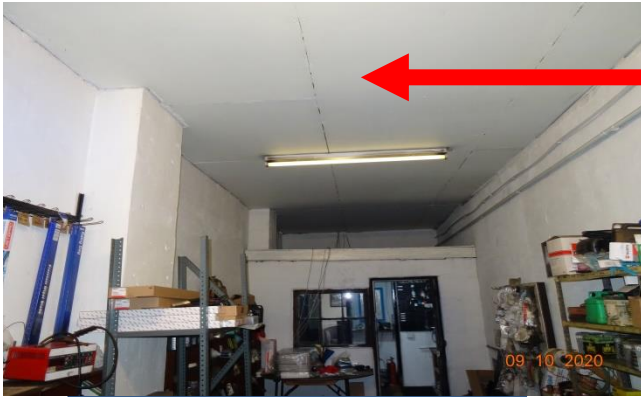
Location Ref 6: Sample TAG/A/S-07- Storeroom - ASBESTOS DETECTED AMOSITE (BROWN ASBESTOS).
