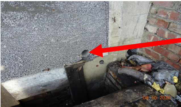
Location Ref 20: Sample TAG/A/S-01- Flue Pipe - ASBESTOS DETECTED CHRYSOTILE (WHITE ASBESTOS).
