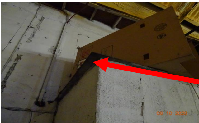
Location Ref 5: Sample TAG/A/S-10- Workshop - ASBESTOS DETECTED CHRYSOTILE (WHITE ASBESTOS).
