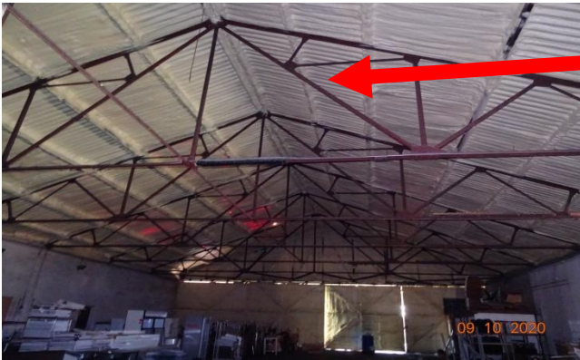
Location Ref 1: Sample TAG/A/S-02- R-Hand Workshop Including Enquires Office - ASBESTOS DETECTED CHRYSOTILE (WHITE ASBESTOS).
