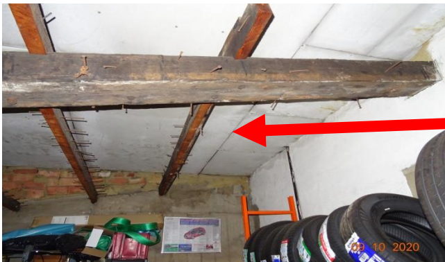
Location Ref 10: Sample TAG/A/S-07- Tyre Storeroom - ASBESTOS DETECTED AMOSITE (BROWN ASBESTOS).
