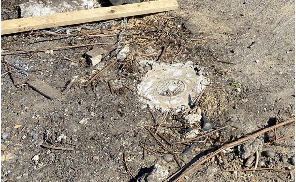
Photo 14: showing WS04 once installed
