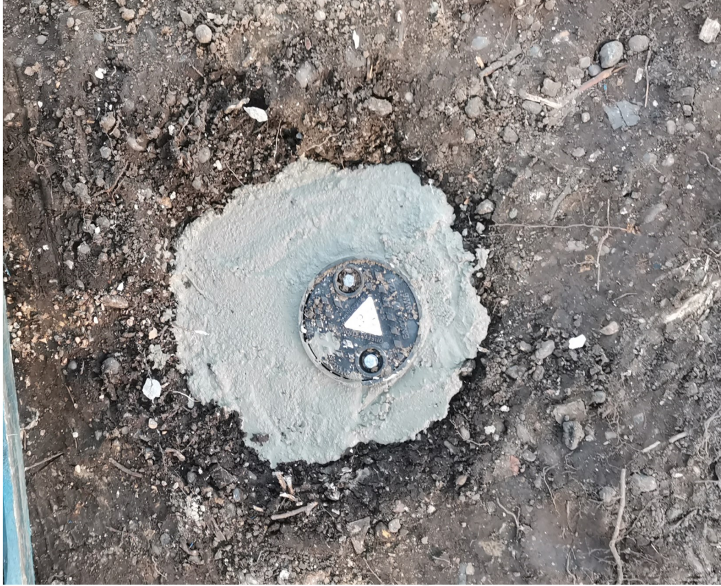
Photo 13: showing WS05 once installed
