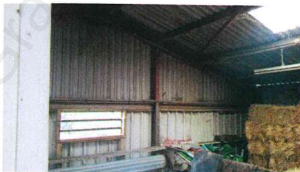
7. Typical steel frame.
