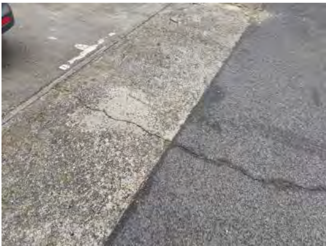
Photo 14—Evidence of cracked concrete in the visitor car parking area
