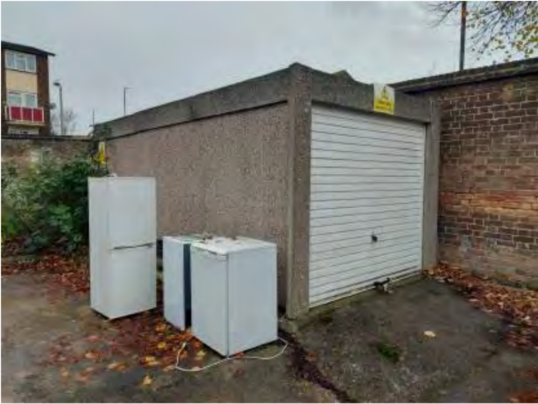
Photo 9—Garage with asbestos roof and stockpile of kitchen appliances
