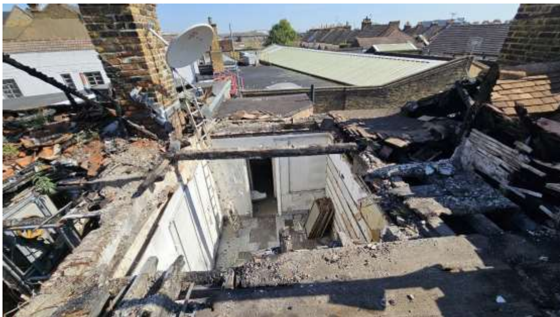
Fig.9: View north from the attic space over the exposed first floor of the property, destroyed by fire.
