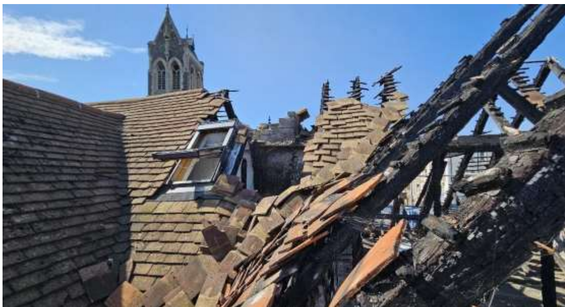
Fig.10: The burnt timbers of no.2 and fire damage extending into no.3.
