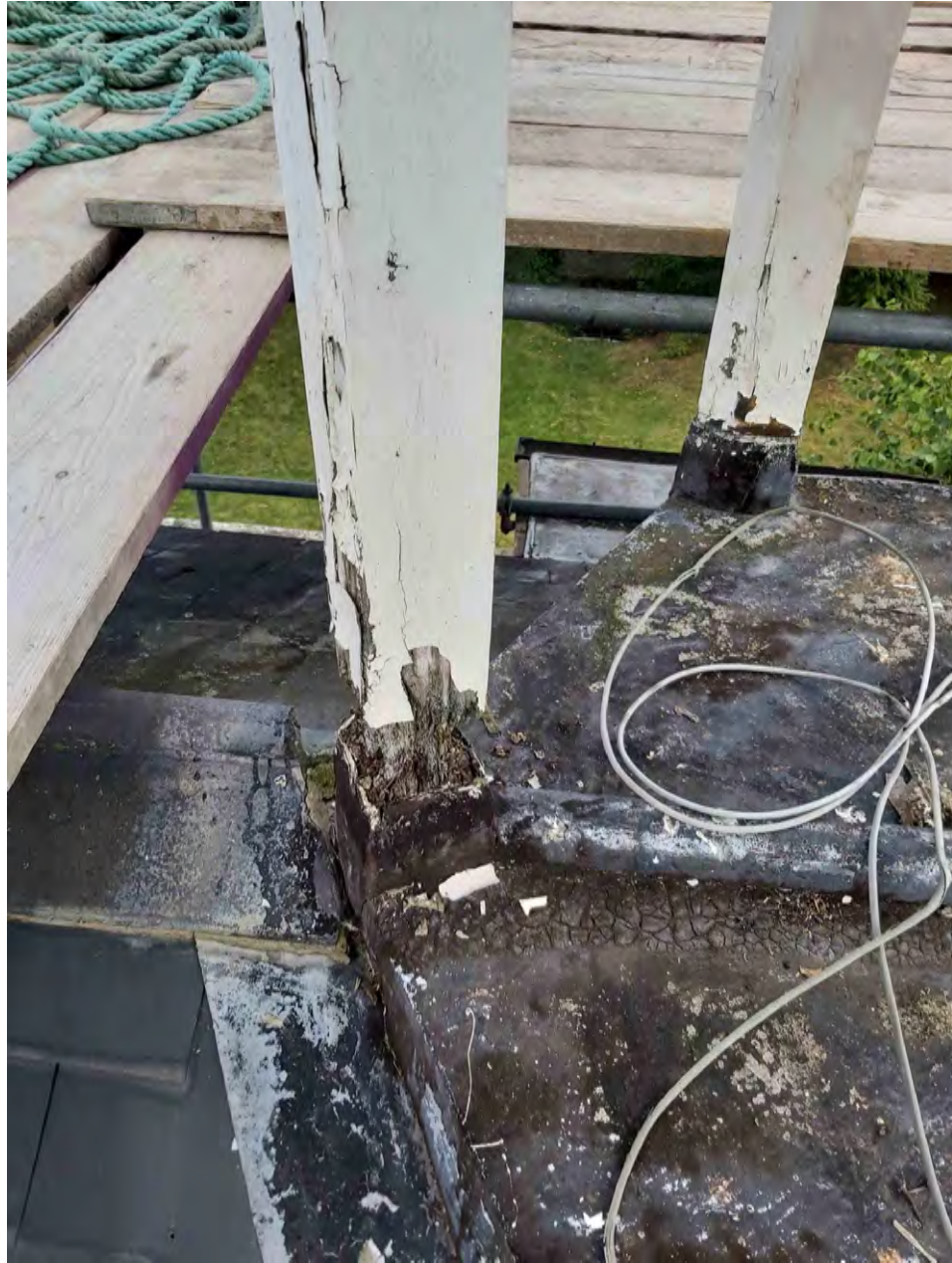
3) Base of cupola post by roof HRFX04. Post is rotten and needs to be replaced. Photograph taken 17/08/2023 by CP
