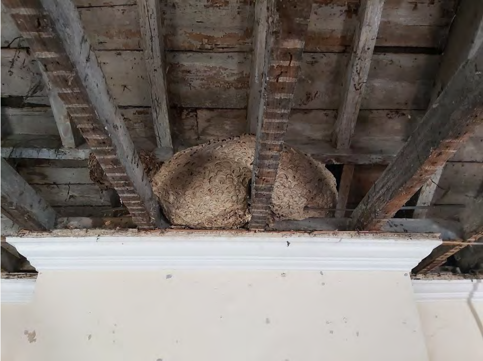
1) Ceiling of HSF06 H1 Classroom looking south Bee/ wasps nest above fireplace. Photograph taken 23/11/2022 by CP
