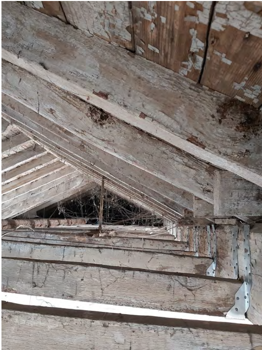
1) Ceiling of HSF06 H1 classroom looking east west Sarking boards have been lime washed . Some boards are showing signs of damp ingress Photograph taken 23/11/2022 by CP
