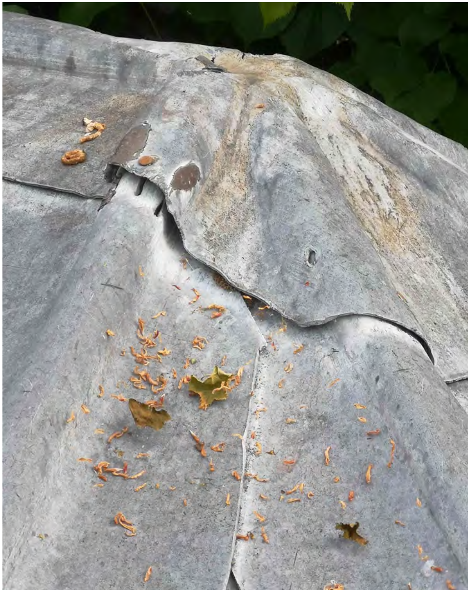
2) Top of roof HRFX07 of HGF0X Library extension looking at the lead ridges. Holes in leadwork where it had been knocked by tree branches over time. Photograph taken 23/05/2023 by BG
