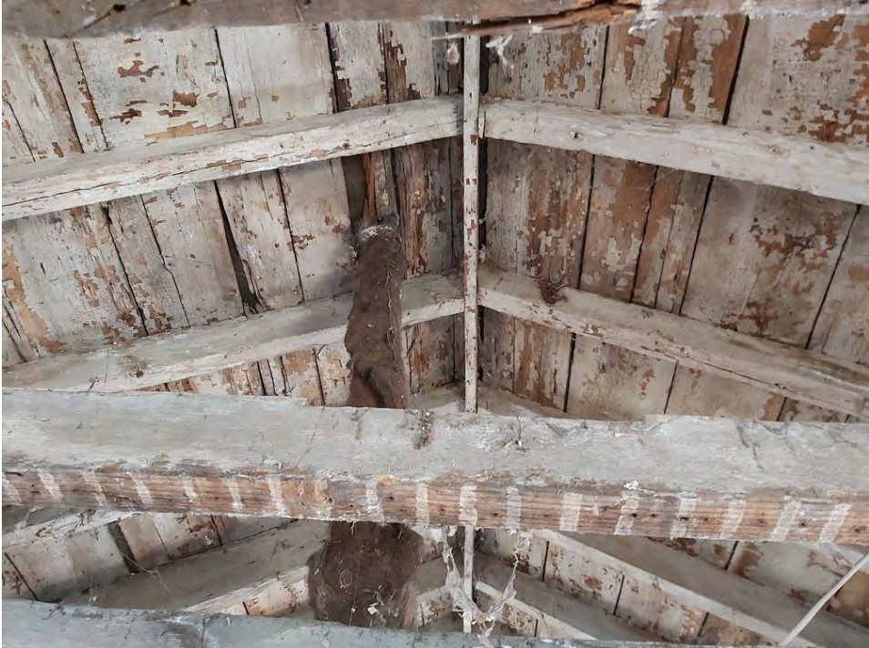
1) Ceiling of HSF06 H1 classroom looking east west Underside of roof RFX02. Gaps between sarking boards. Some are rotten and damp coming in from above. Photograph taken 23/11/2022 by CP
