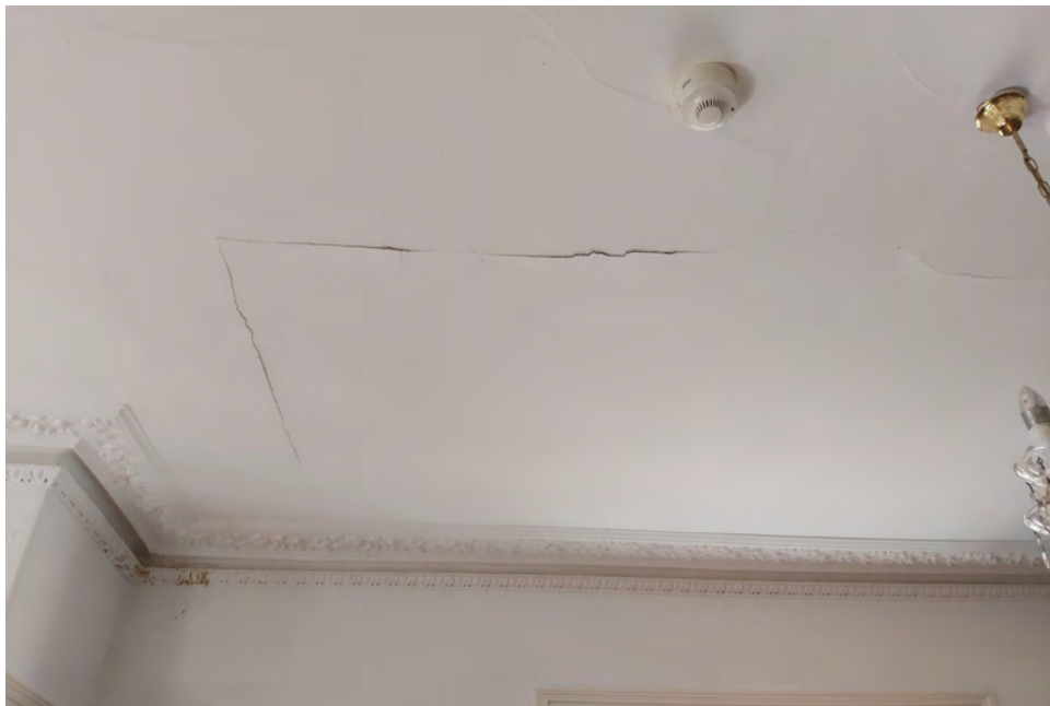
2) Ceiling of HGFX0X Library extension looking east west Cracks appearing around the plasterboard ceiling Photograph taken 04/05/2023 by CP
