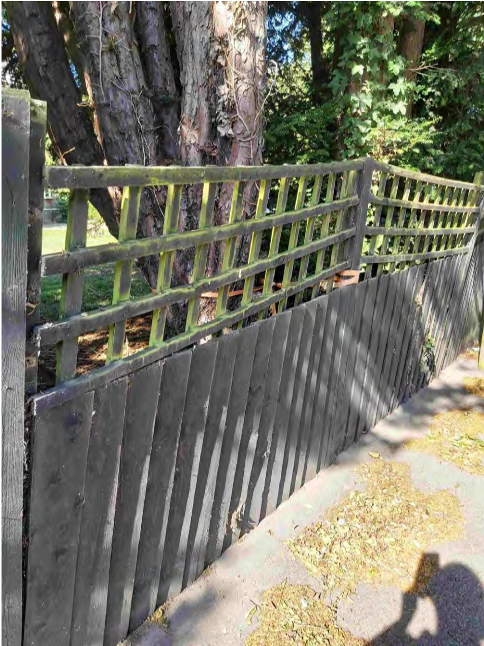
9) Front boundary fence facing Gravesend Road between driveway gates. Close boarded timber fence with open trellis above. The fence posts are rotting. The fence has been fixed down to the top of a low brick wall that straddles the tunnel below. Photograph taken 16/08/2023 by CP
