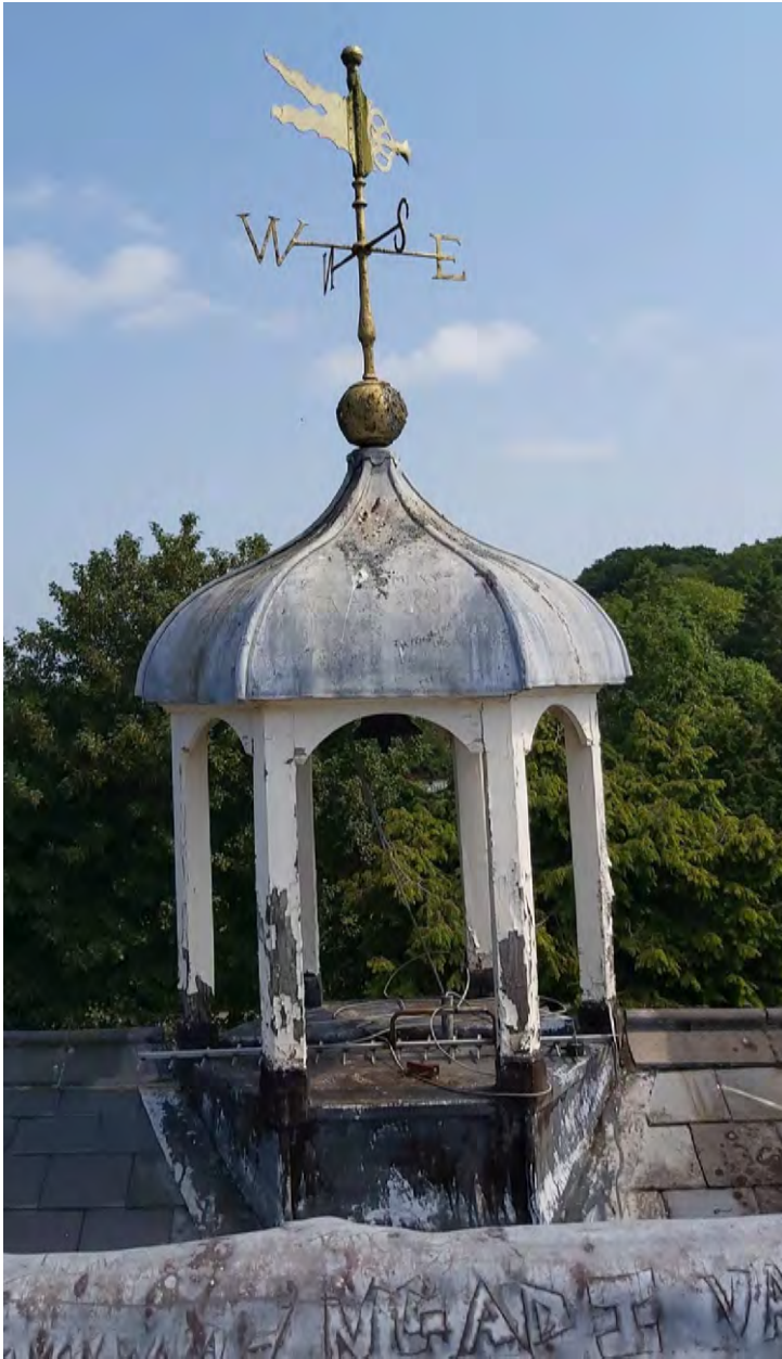
3) Cupola HCPX01 looking north. Some of the posts are rotten, paintwork has cracked allowing water ingress. Cupola has twisted. Photograph taken 09/06/2023 by CP
