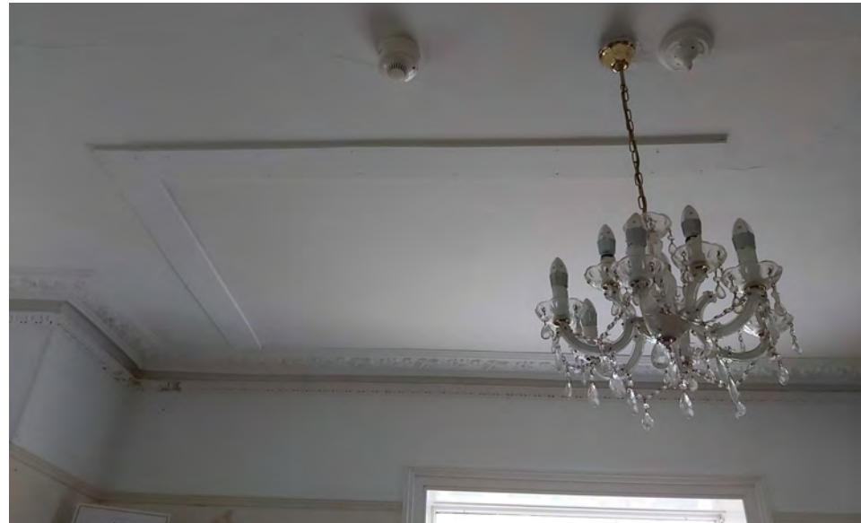
2) Ceiling of HGFX0X Library extension looking east west Temporary repair has been carried out. Photograph taken 04/08/2023 by CP
