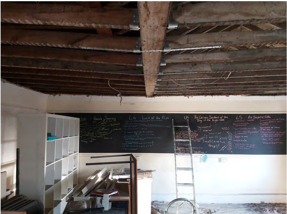
1) Ceiling of HSFX06 H1 classroom looking east After ceiling came down on the advice of the SE straps were fixed to underside of main beam. Photograph taken 23/11/2022 by CP
