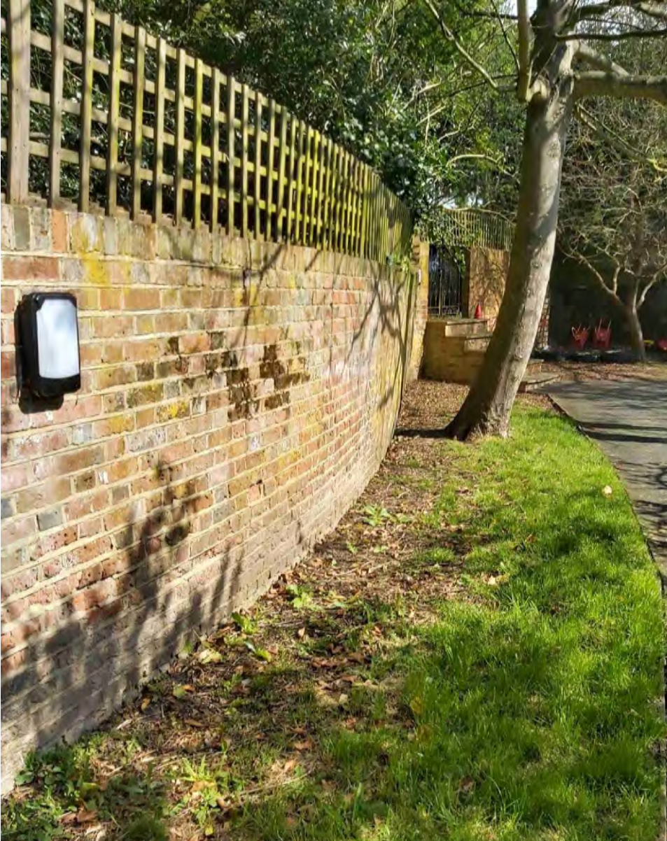
4) Garden wall between front drive and orchard. Wall is bulging. Photograph taken 03/05/2023 by CP
