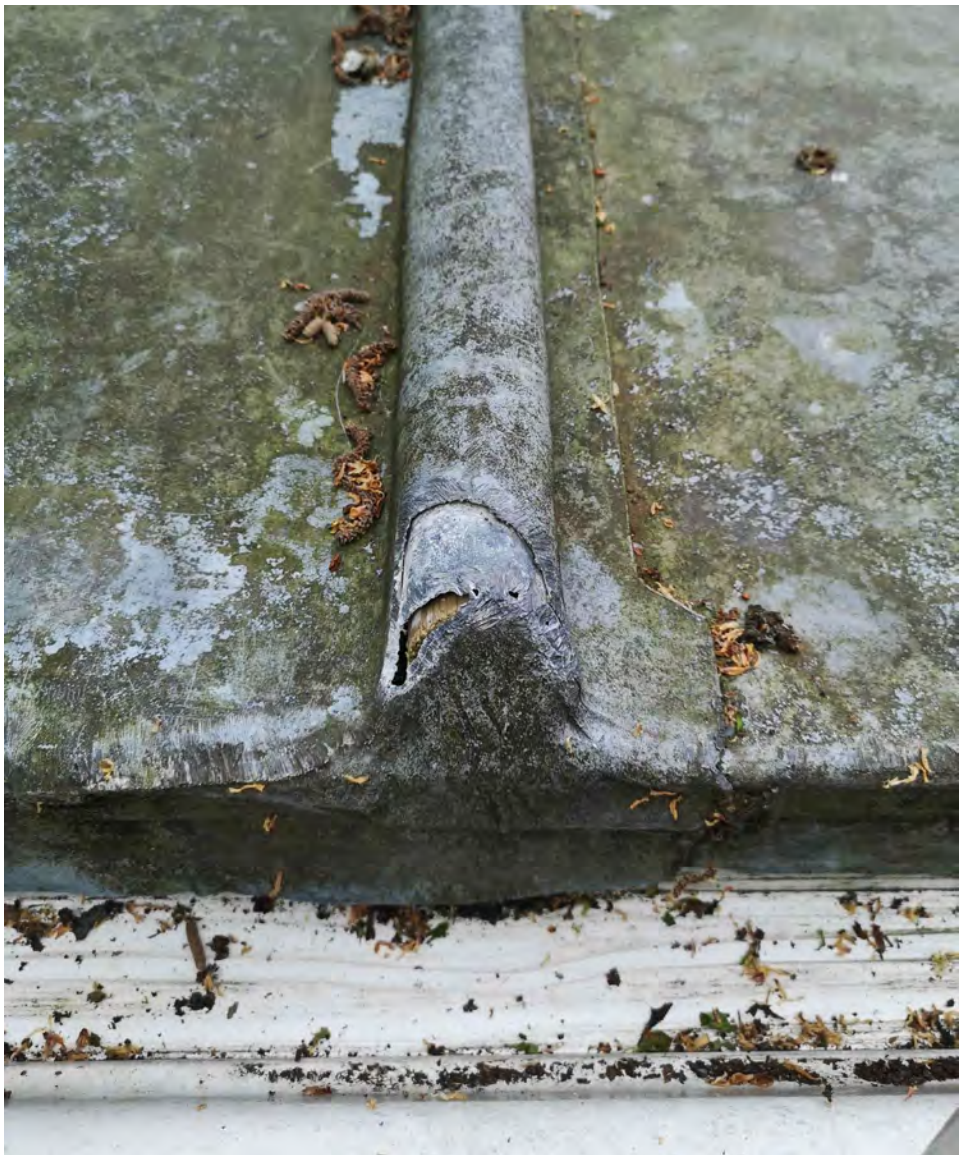
2) Roof HRFX08 Library extension looking east west Lead roof has been nibbled by squirrels Photograph taken 23/05/2023 by BG
