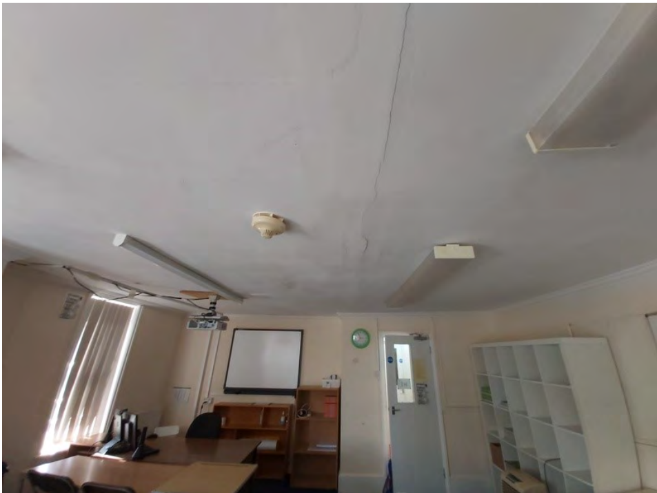
1) Ceiling of HSFX06 H1 classroom looking west Ceiling shows signs of cracking , sagging and previous repairs. Photograph taken 01/08/2022 by CP
