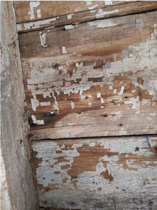
1) Underside of roof HRF02 of HSF06 H1 class-room looking at the sarking boards. Sarking boards showing signs of water ingress coming in from above. Photograph taken 23/11/2022 by CP
