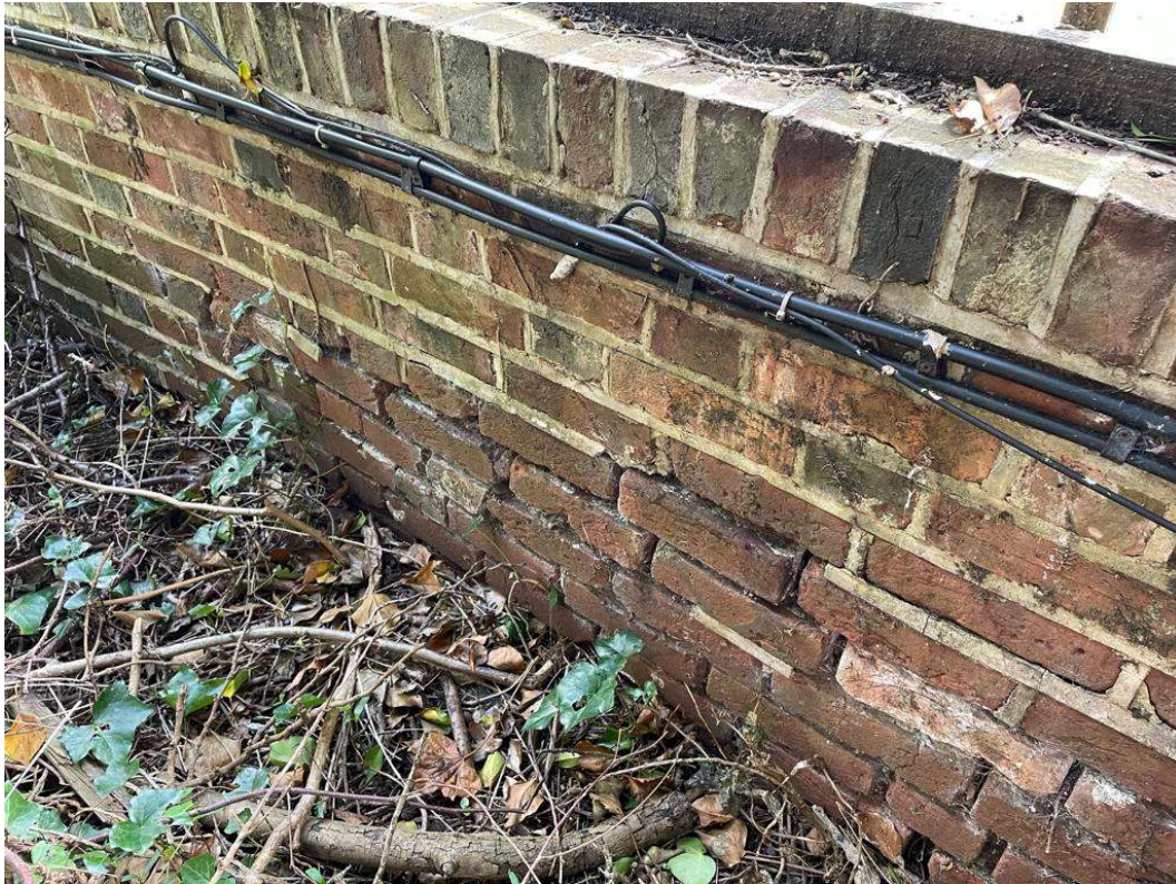
View on mortar loss to rear face of wall near to vertical crack
