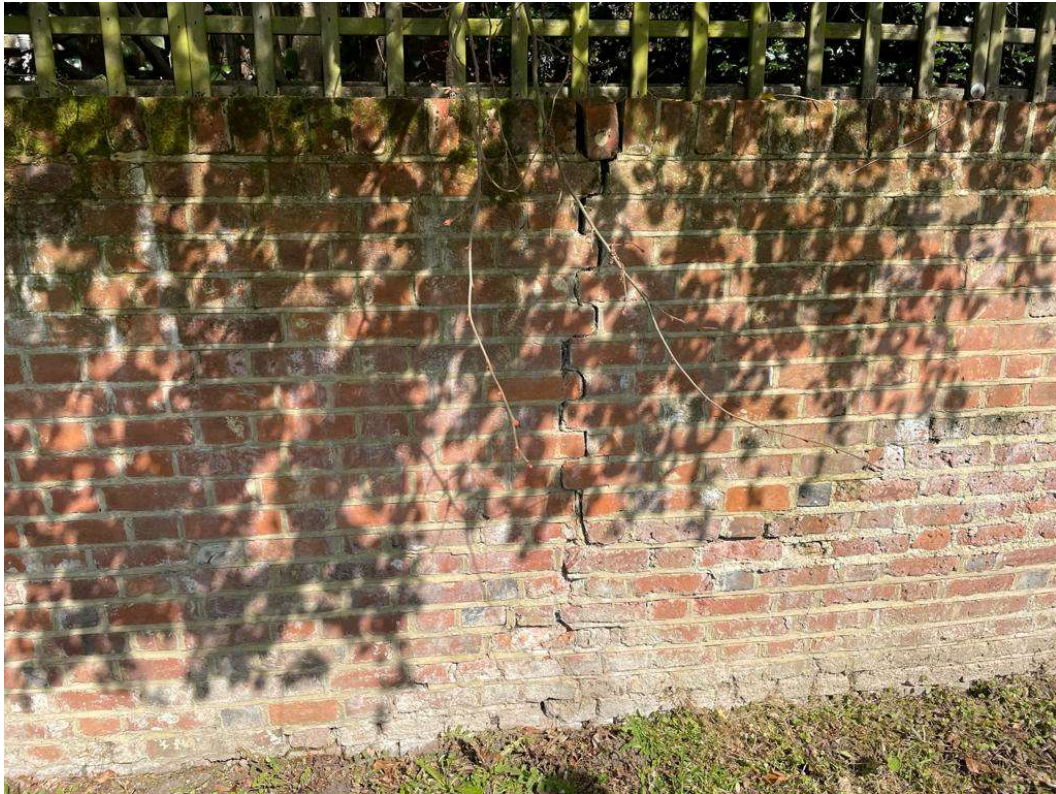
View on tapering vertical crack in retaining wall
