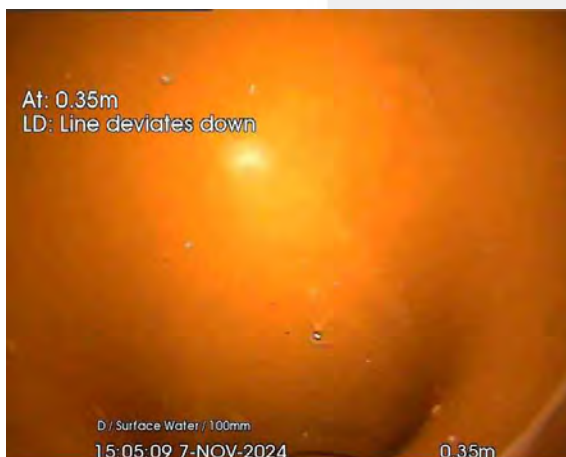
361.jpg, 00:00:05, 0.35 m Line deviates down
