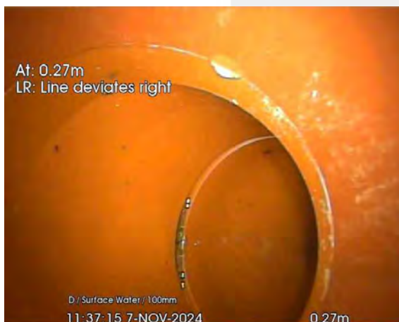
233.jpg, 00:00:06, 0.27 m Line deviates right
