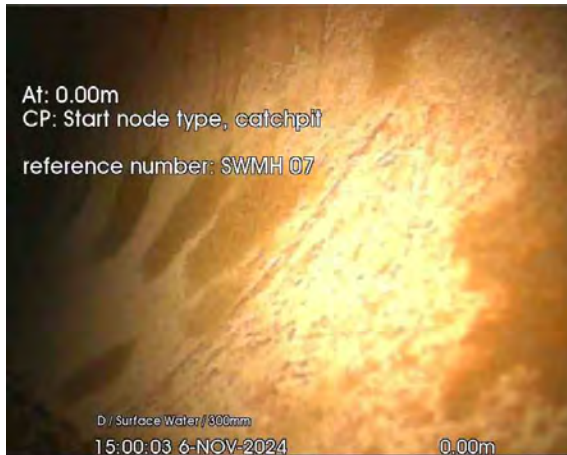
103.jpg, 00:00:02, 0.00 m Start node, catchpit, reference: SWMH 07
