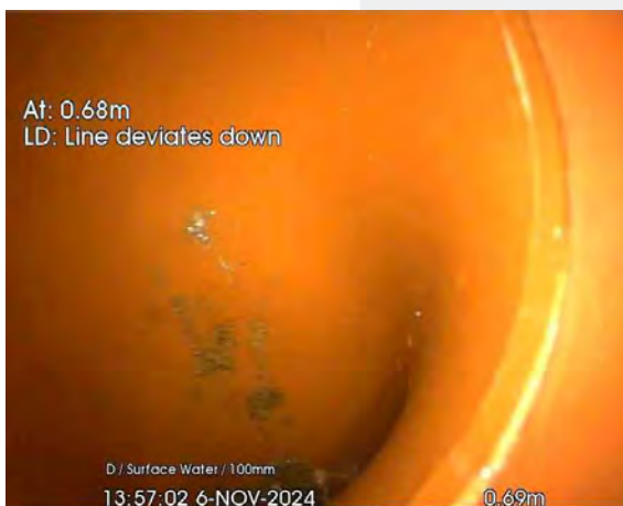
40.jpg, 00:00:09, 0.69 m Line deviates down
