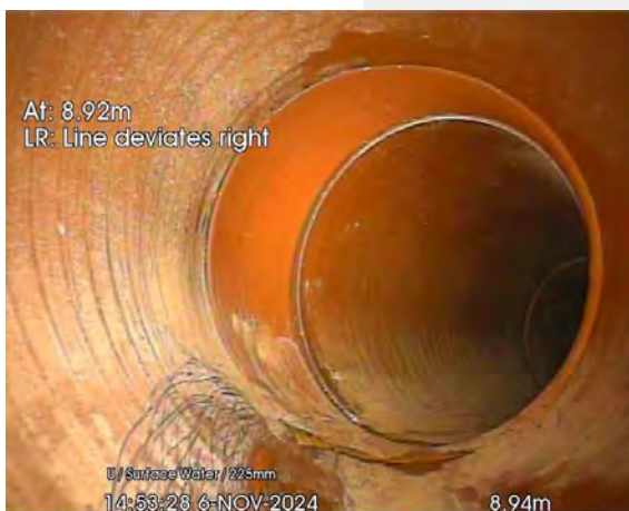
101.jpg, 00:00:46, 8.94 m Line deviates right
