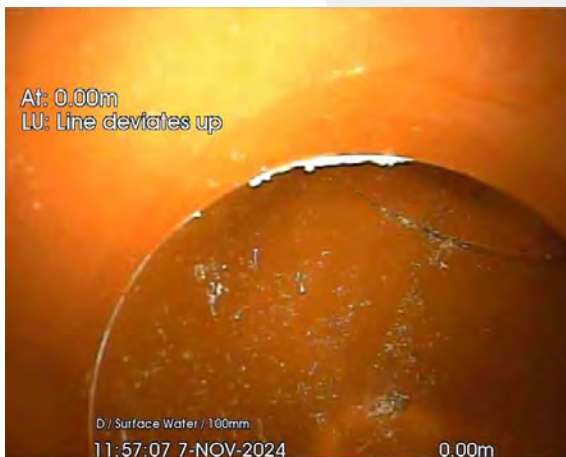
253.jpg, 00:00:06, 0.00 m Line deviates up
