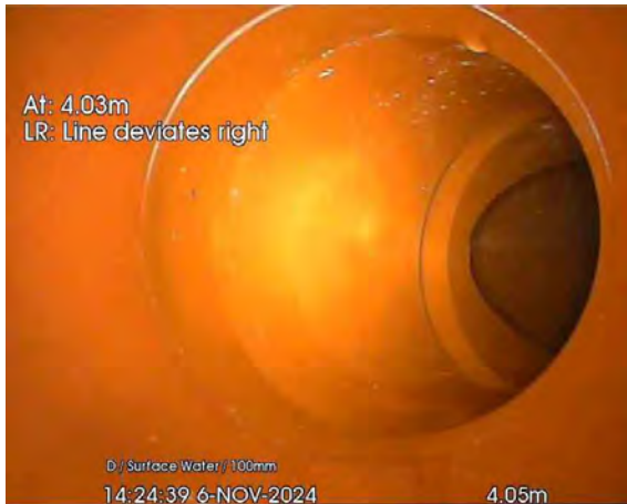
73.jpg, 00:00:32, 4.07 m Line deviates right
