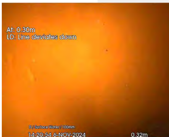
66.jpg, 00:00:09, 0.34 m Line deviates down
