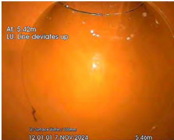
259.jpg, 00:00:28, 5.46 m Line deviates up
