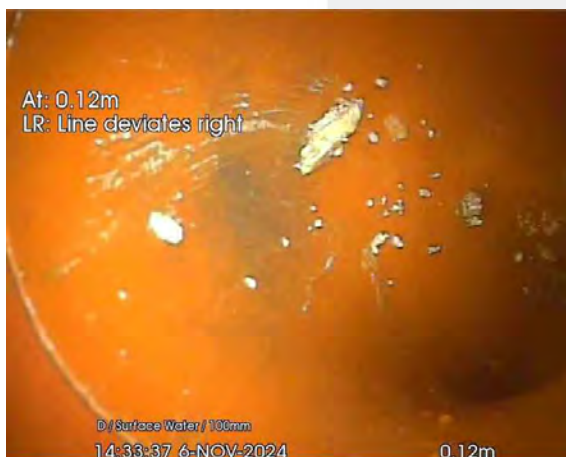
82.jpg, 00:00:05, 0.12 m Line deviates right
