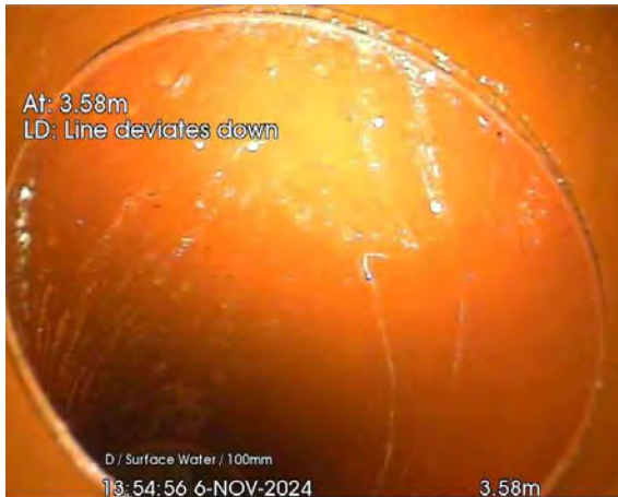
36.jpg, 00:00:28, 3.58 m Line deviates down
