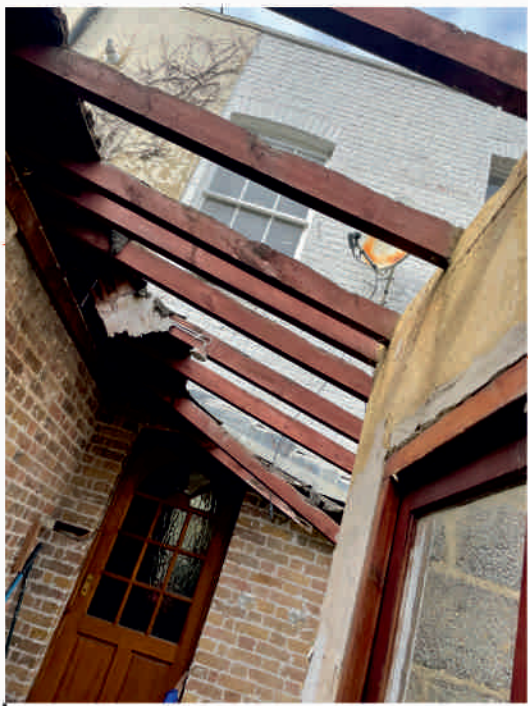
PHOTOGRAPH 7, Showing derelict rear addition
