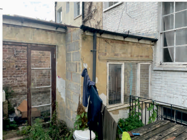
PHOTOGRAPH 2 Showing extension at first floor it can be seen it is in poor condition with a collapsed roof. The walls are single skin rendered block work and non-original. It also shows that existing facing brickwork to the rear has been painted white.
