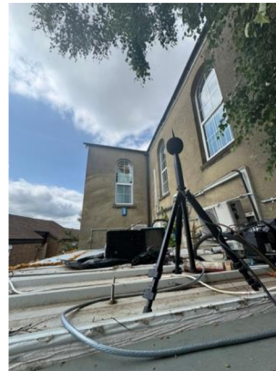
Figure 2 – South Chiller & AC Units
