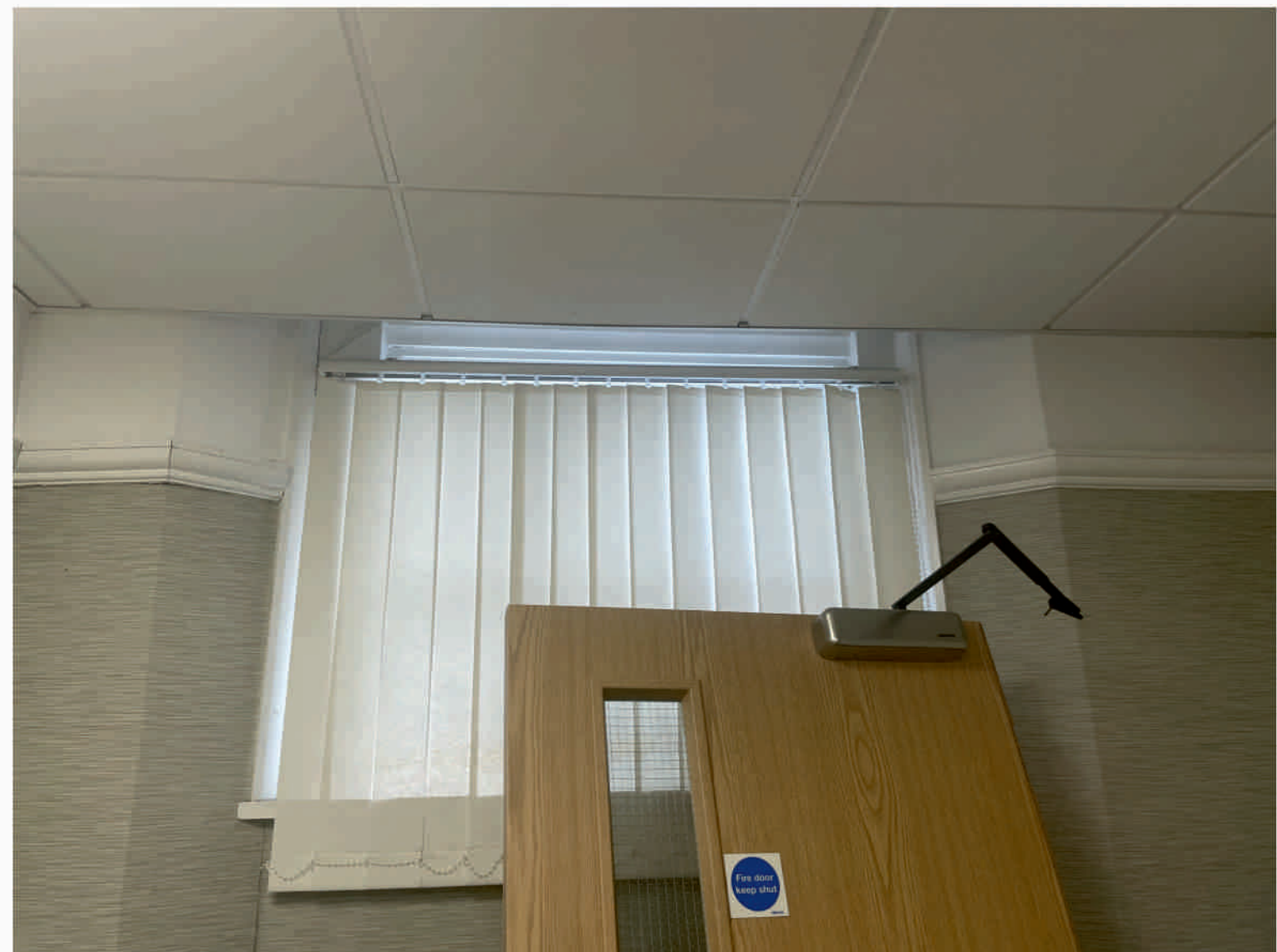
ROOM 6 - Original top hung plain window at high level over roof of lower ground floor level. original picture rail to remain. Not suspended ceiling. Checked void which is used for services cornice damaged.
