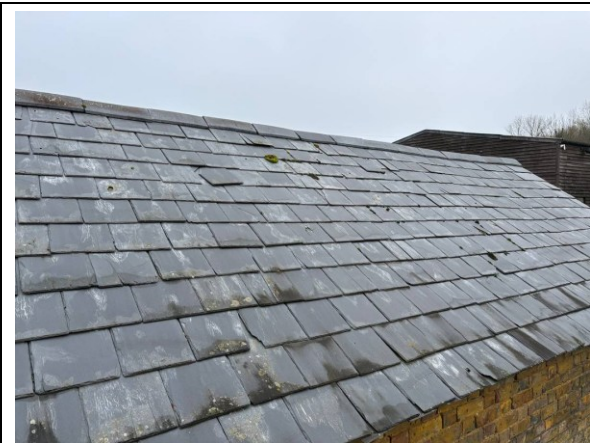
Photo 7: Building B1, lifted/slipped roof tiles
