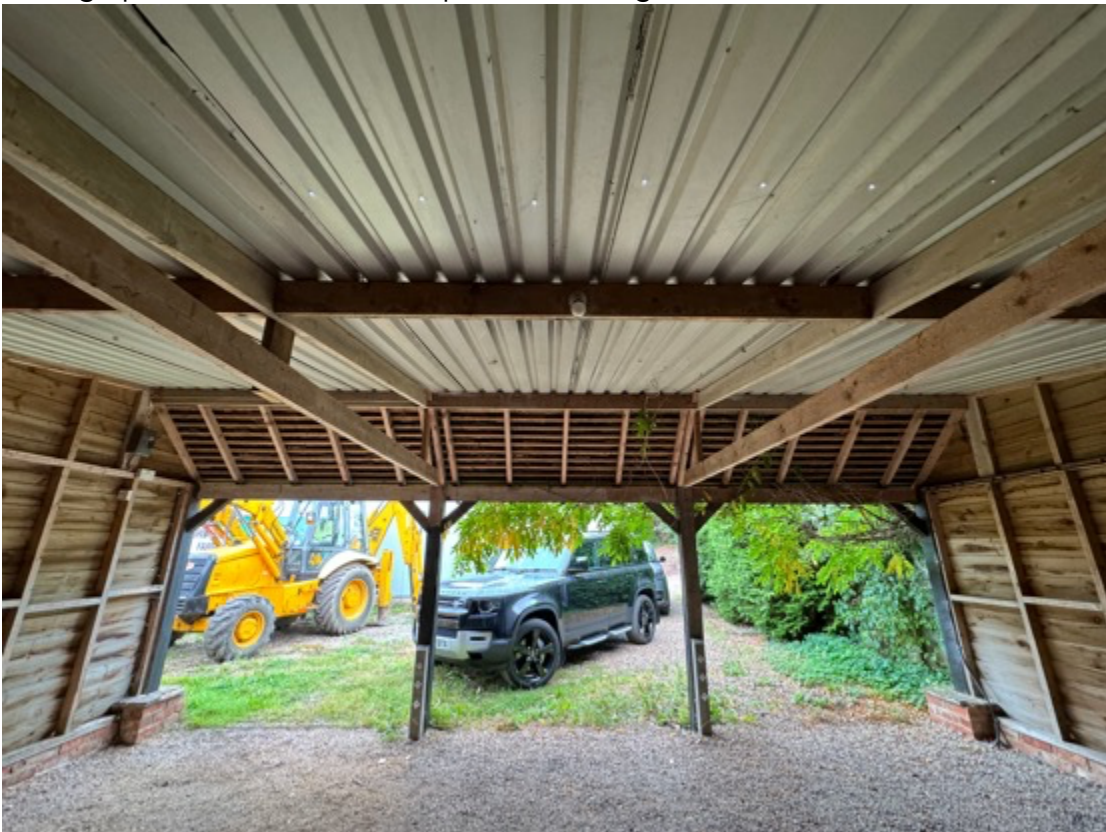
Photograph 12: Interior of the carport, illustrating small, front tiled roof area with no membrane
