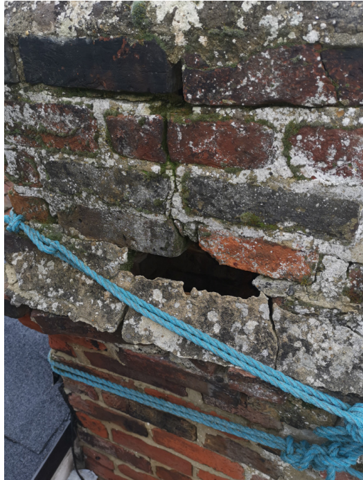
P004 – southern face of chimney indicating cracking and apperture through to internal flue
