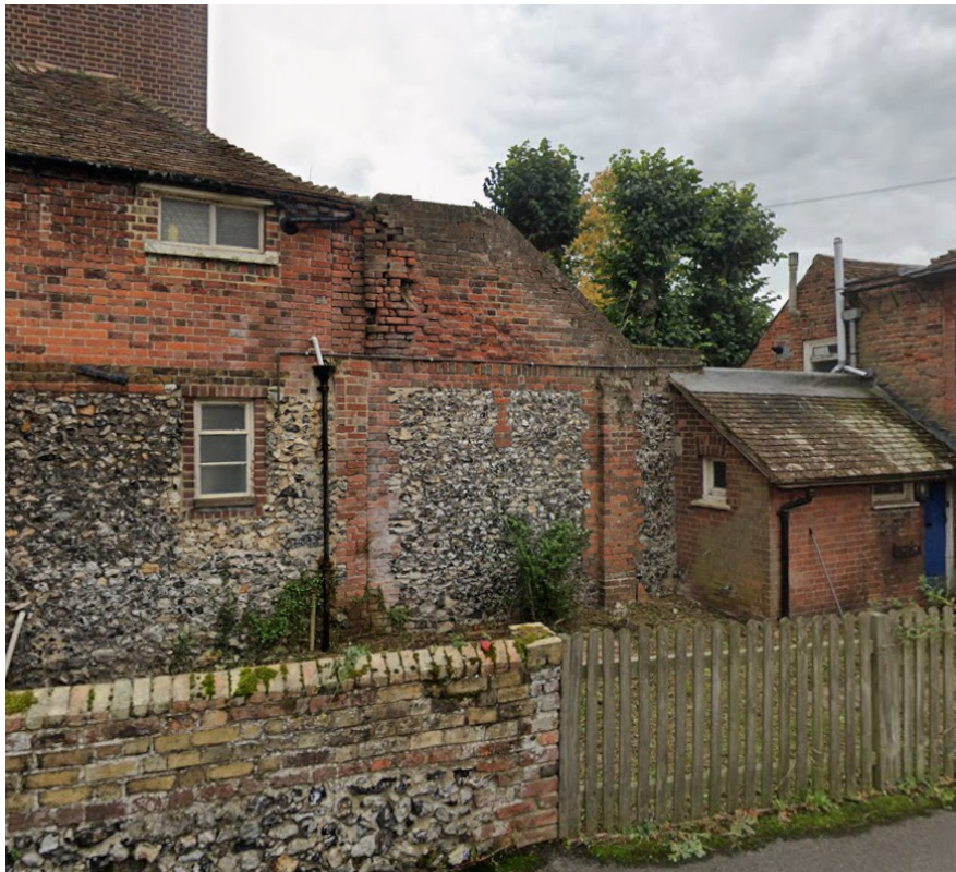
P001 Parapet wall and failed external corbel from Crutches Lane
