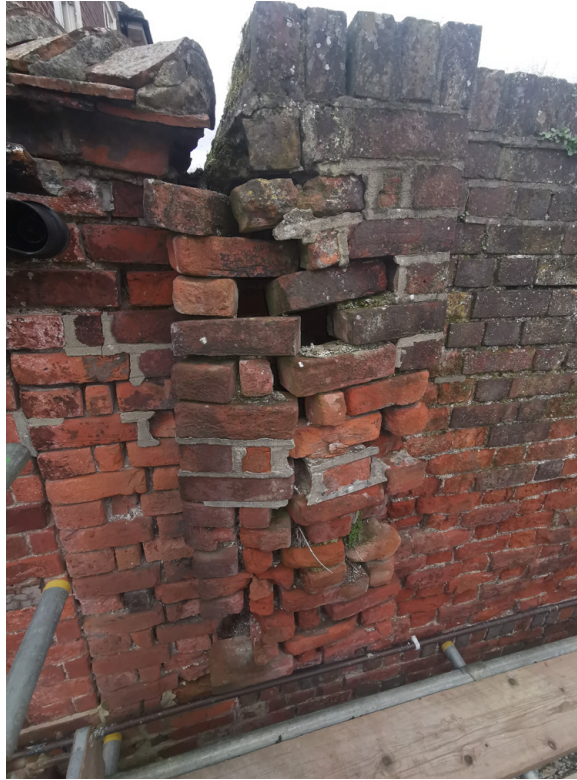
P002 – close up of failed corbel
