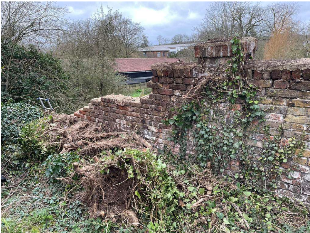
View of failed wall and surviving but weak and unstable boundary wall
