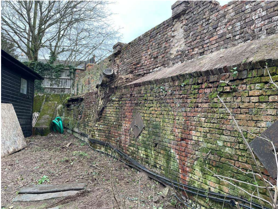
View along eastern wall looking to north showing damage to boundary and retaining walls
