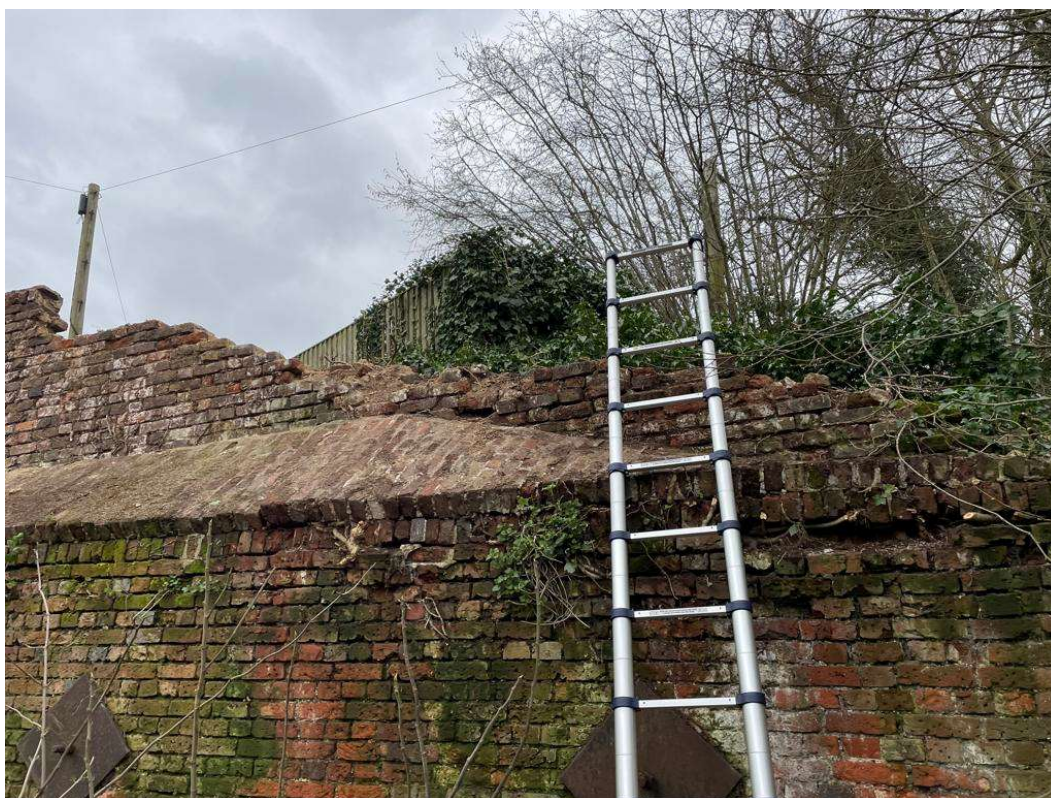
View on unprotected edge from lower ground level
