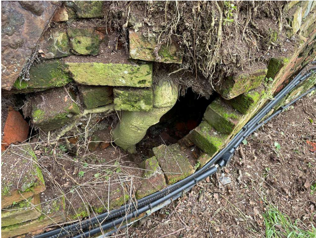
Detailed view on tree root damage and penetration into wall brickwork
