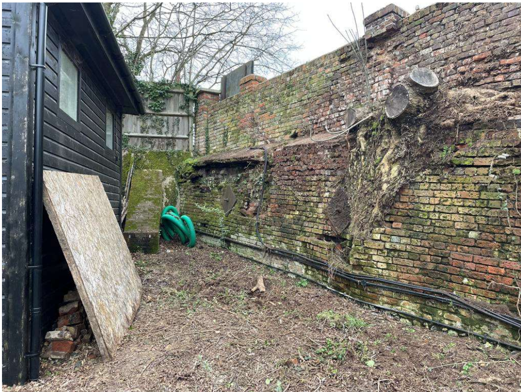
View on northern end of east wall showing proximity to kindergarten, brick loss, sycamore tree roots and damage caused
