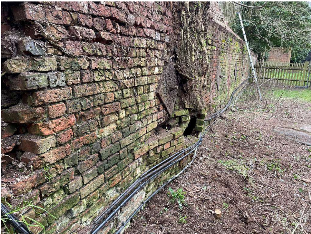
View on lower tree roots showing damage to retaining wall brickwork
