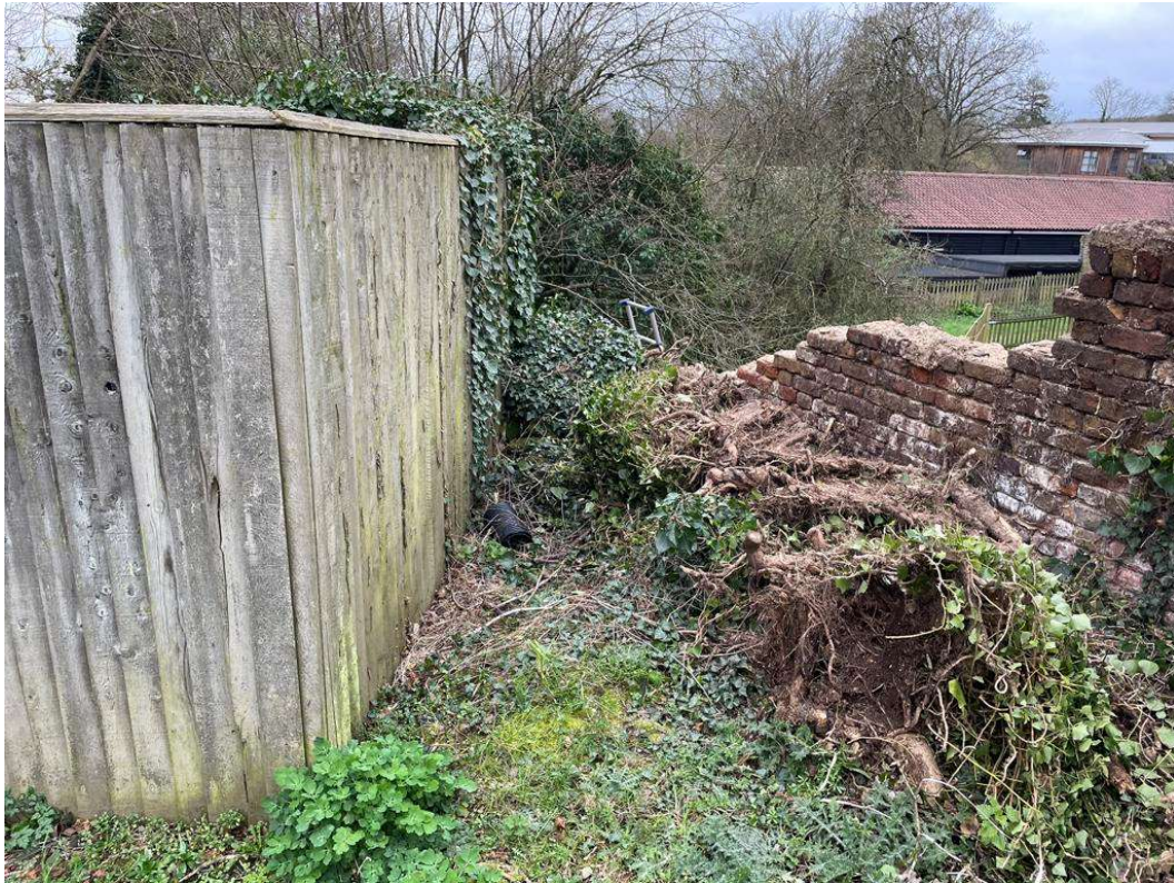
View of failed boundary wall at upper level showing lack of restriction and safety protection to any persons
