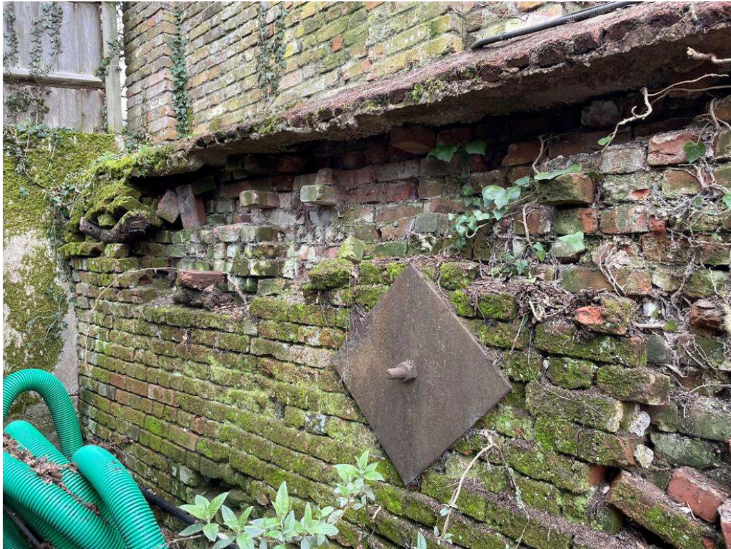
Close up view of failed brickwork also showing ground anchor
