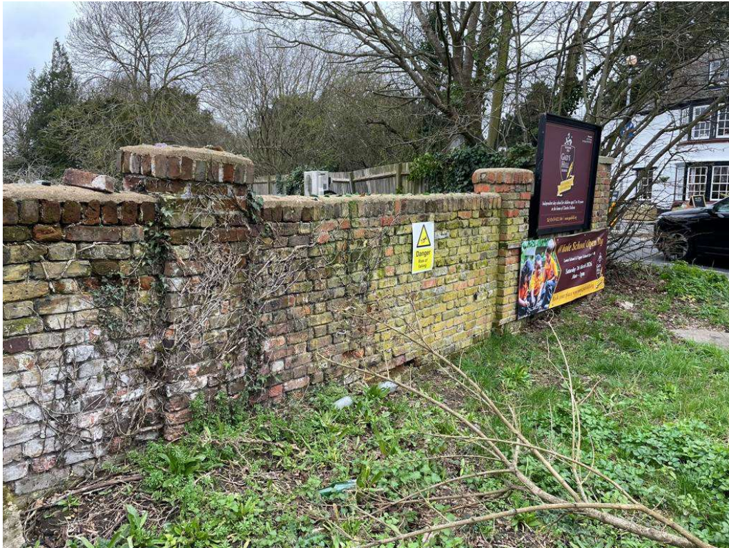
View on upper level boundary wall showing short length of undamaged wall
