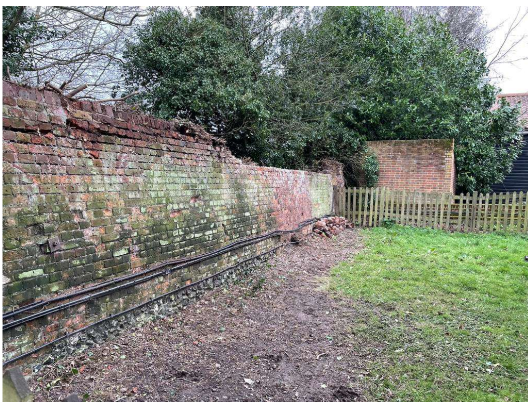
View on length of non-retaining boundary wall at low level towards the Pavillion showing damage to top of wall and outward leaning at mid-distance
