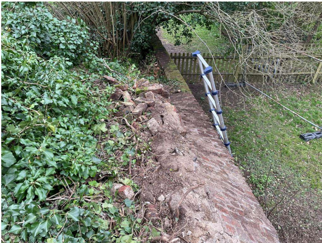
View on unprotected edge where boundary wall has failed
